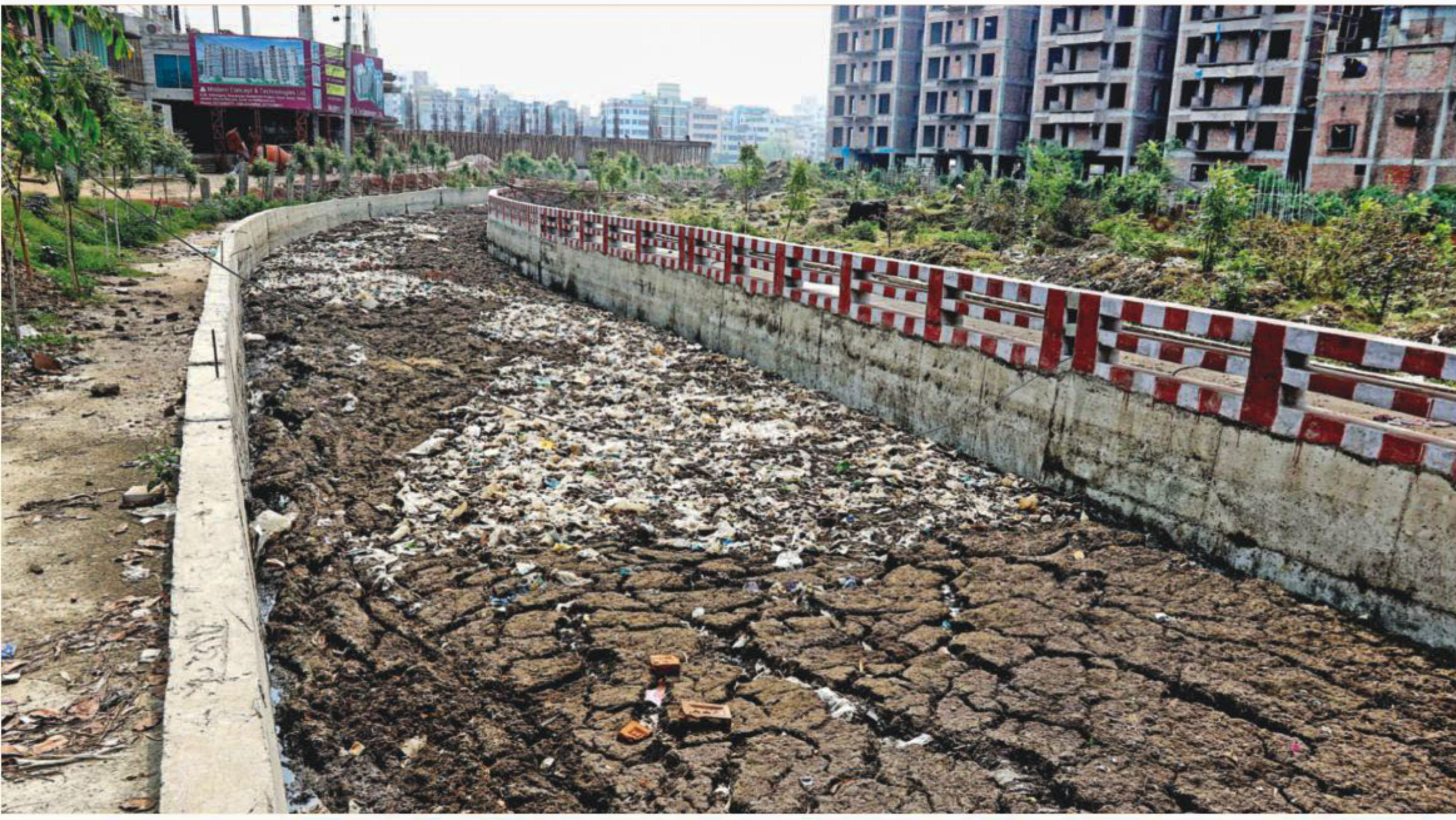
Within just one year, almost a half-kilometre stretch of the newly rebuilt drainage canal, known as Rayerbazar Khal, has been completely clogged with a four or five feet deep layer of sludge. Locals said the situation had resulted from a lack of maintenance in the absence of the elected public representatives. The photo was taken recently.
