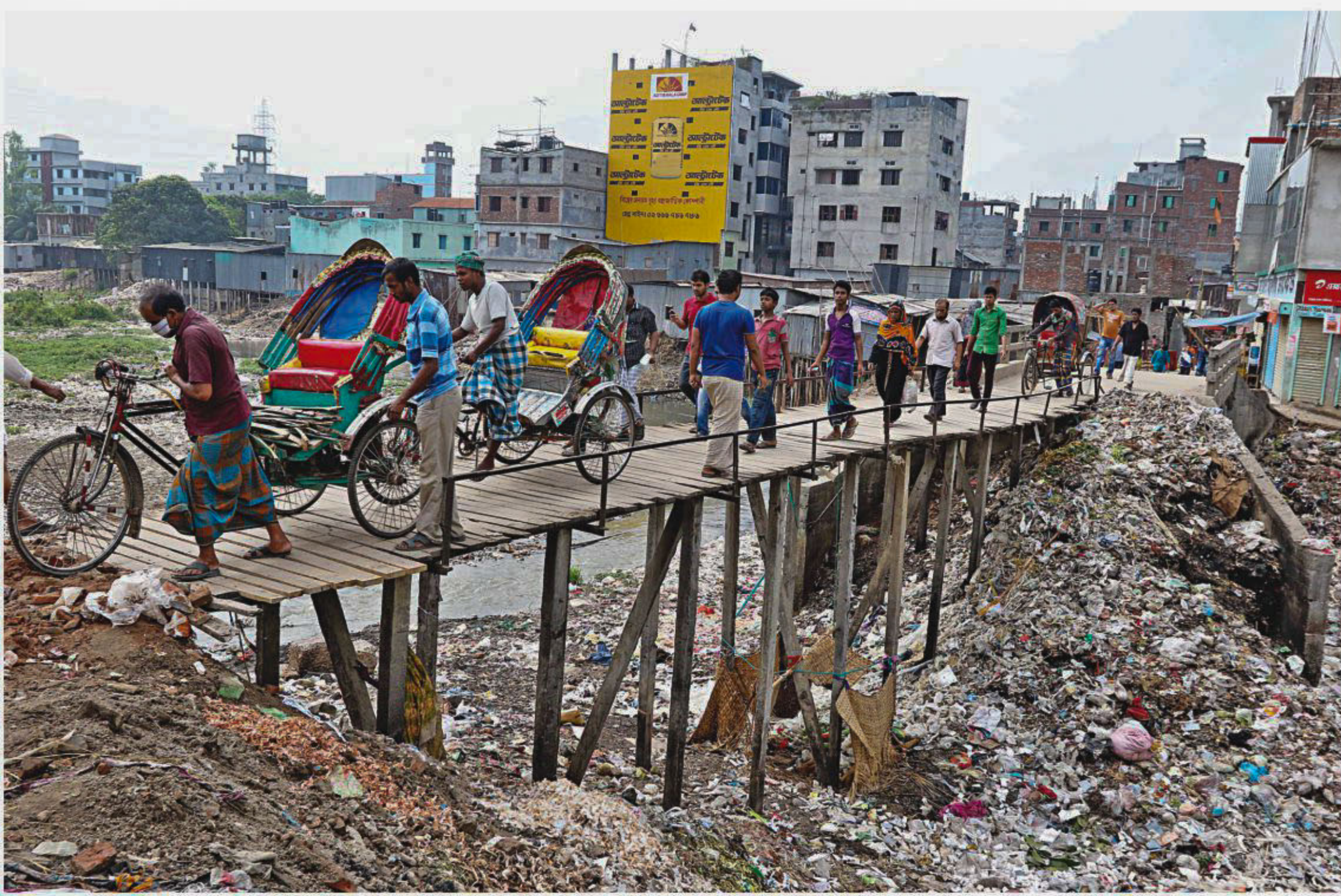
People are using this risky wooden structure to commute between Lalbagh and Purba Rasulpur of the capital while a half-built concrete bridge has not seen completion in the last six years. The photo was taken on Thursday.
