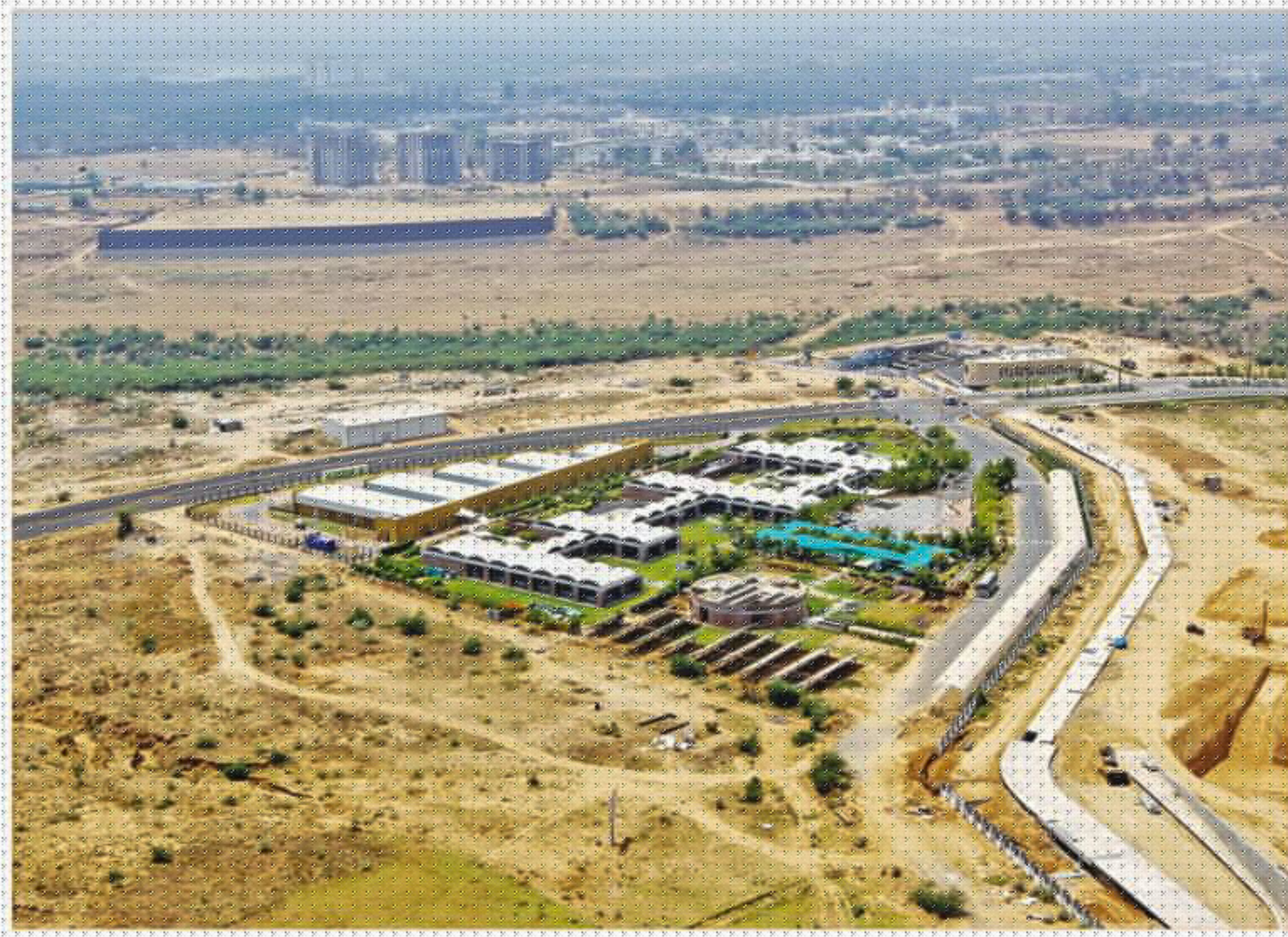
An aerial view of a site under construction at the Gujarat International Finance Tec-City at Gandhinagar in Gujarat, India.
