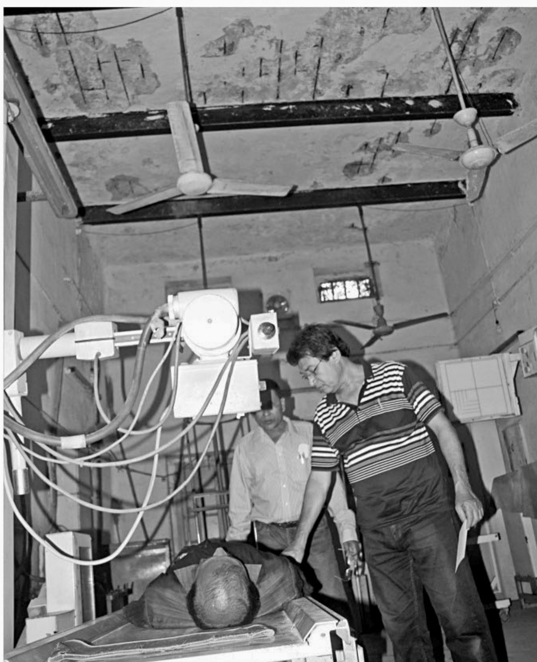
A patient undergoes an x-ray examination in a dilapidated room of the century-old Barisal General Hospital on Wednesday, half an hour after plaster fell off the ceiling injuring a patient and a staff. The soggy, flaking walls and ceilings are also damaging the expensive medical equipment but the Public Works Department and Department of Public Health Engineering (DPHE) are exchanging blames over the hospital's maintenance and renovation.
