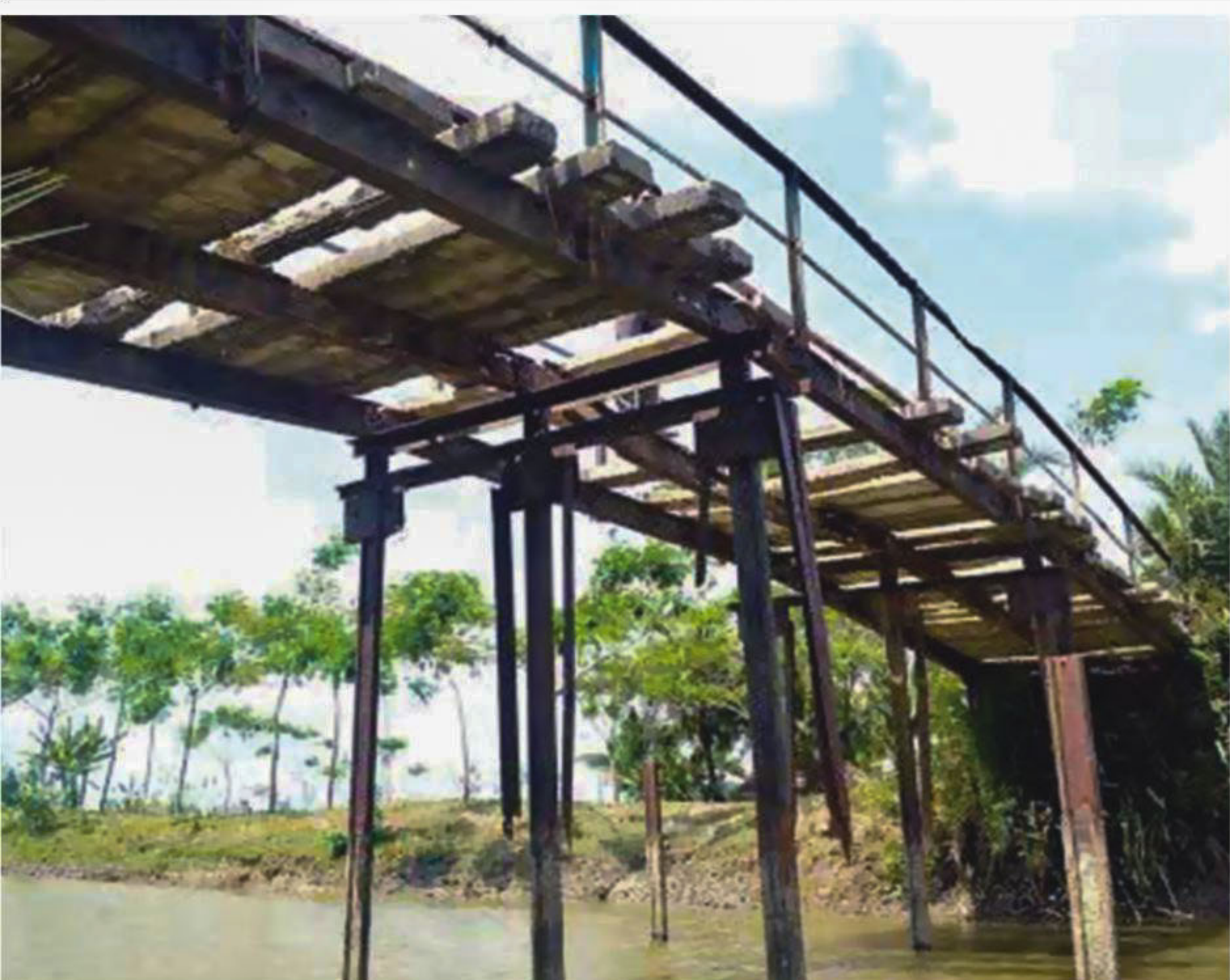
This iron bridge over Dora canal in Dhulasar union of Kalapara upazila under Patuakhali district has remained virtually unusable for the last two years, much to the sufferings of around 8,000 people of six villages.
