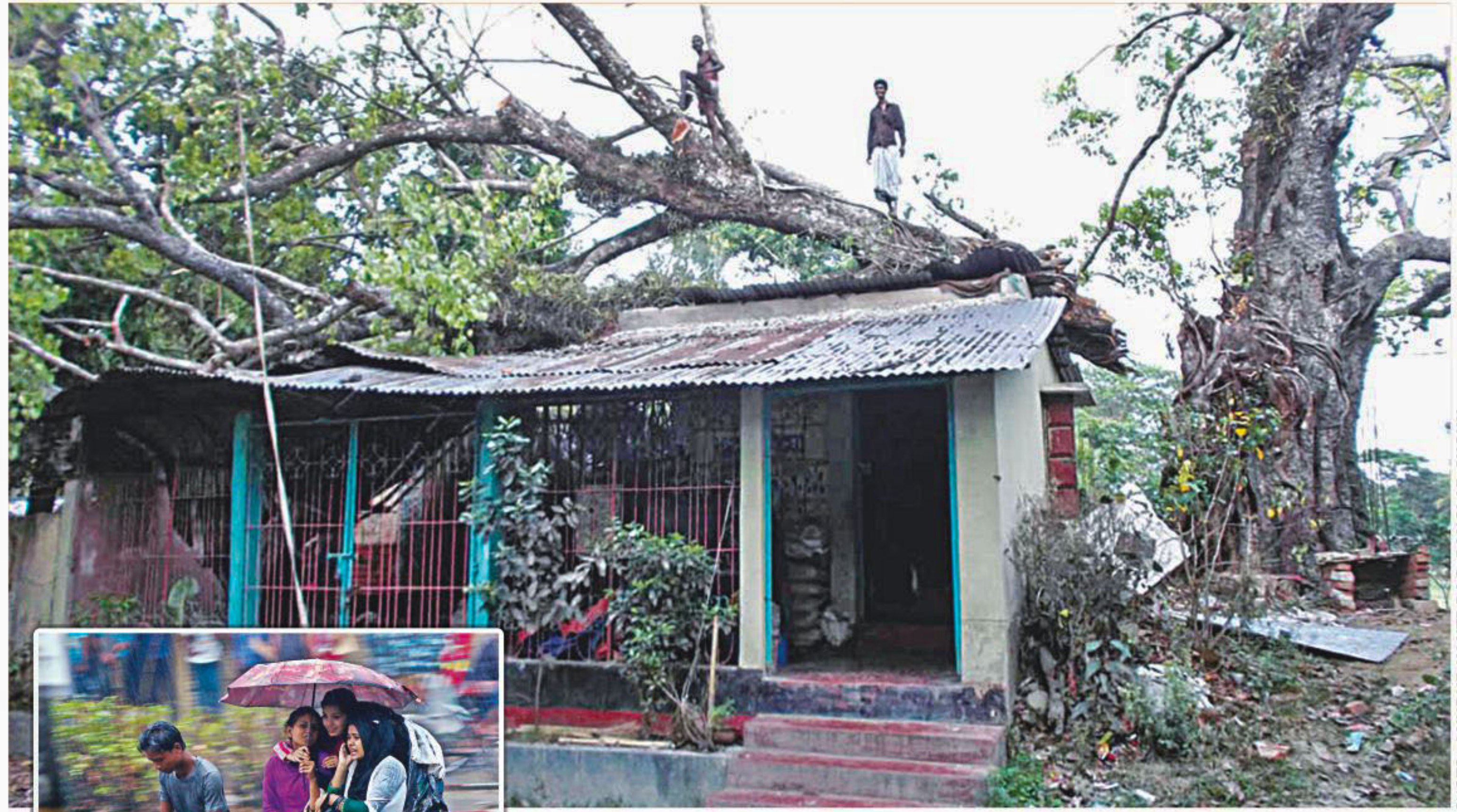
A house that partially survived the fall of a heavy tree branch, among the ravages of a storm, which torn through Mirsarai of Chittagong, while Chittagong city, inset, is drenched by a sudden downpour yesterday, signalling the arrival of the violent nor'easter season.
