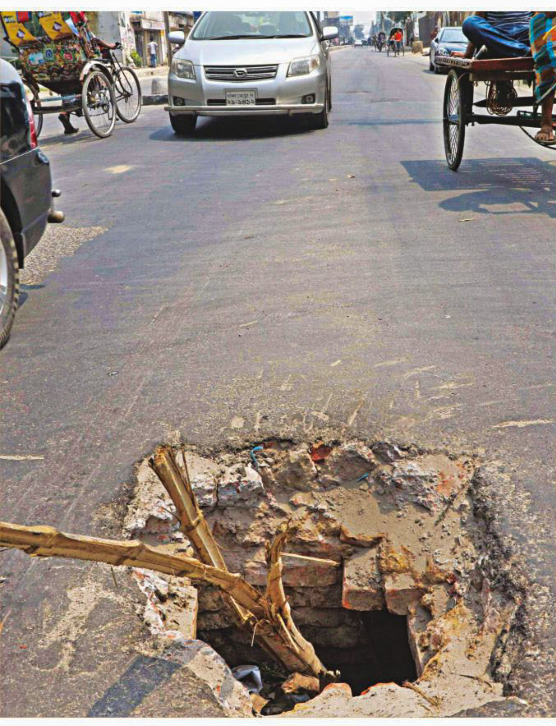
Motorists speed past this large drainage opening barely aware of the danger, especially when a bamboo pole is the only thing to warn them, on Tejgaon Link Road in the capital. The photo was taken on Friday.
