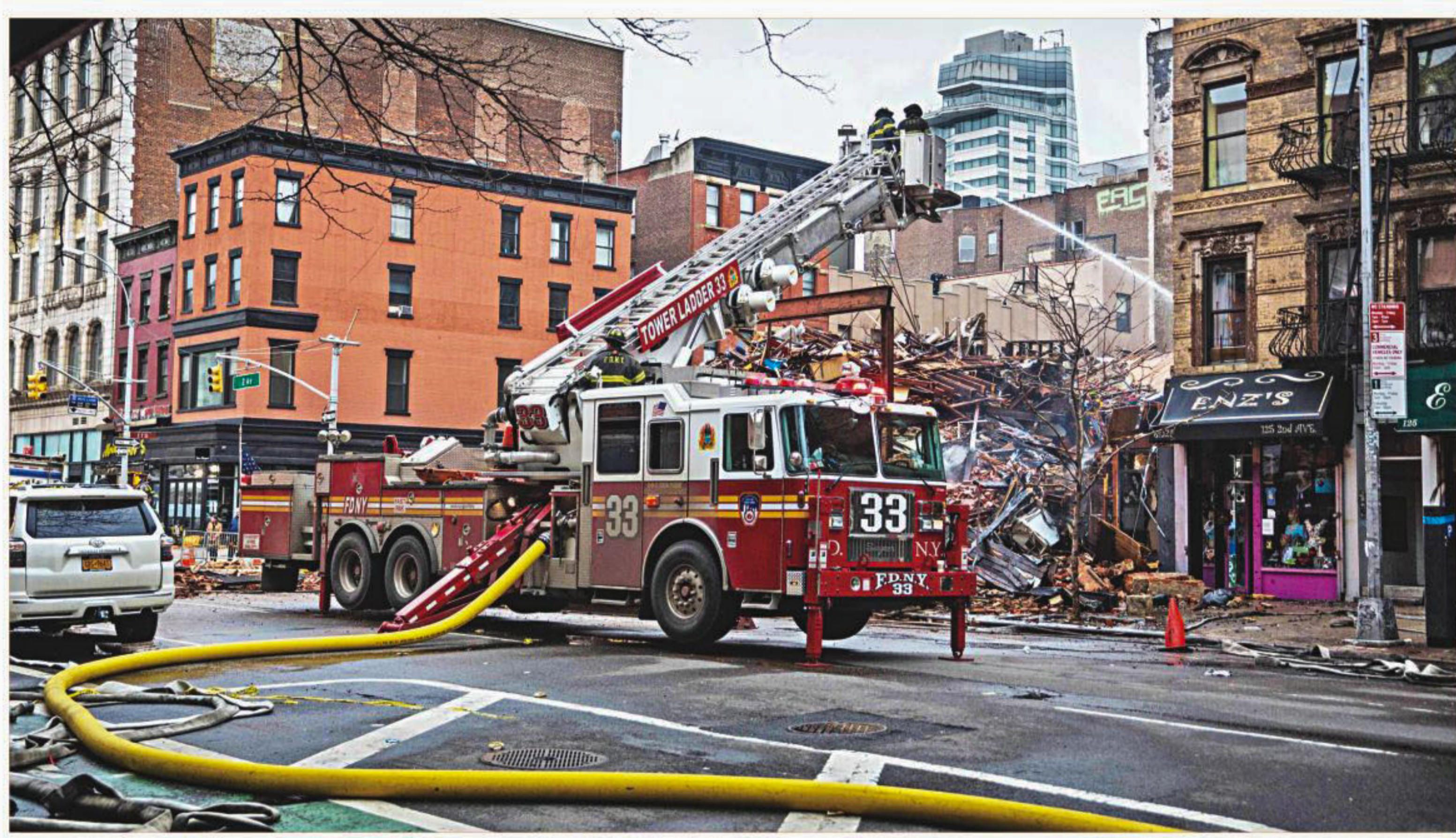
Firefighters continue to hose down the site of a fire incident that caused the collapse of two buildings and damage to two other buildings a day after the blaze took place in New York City. At least two people are missing and over a dozen injured in the accident.
