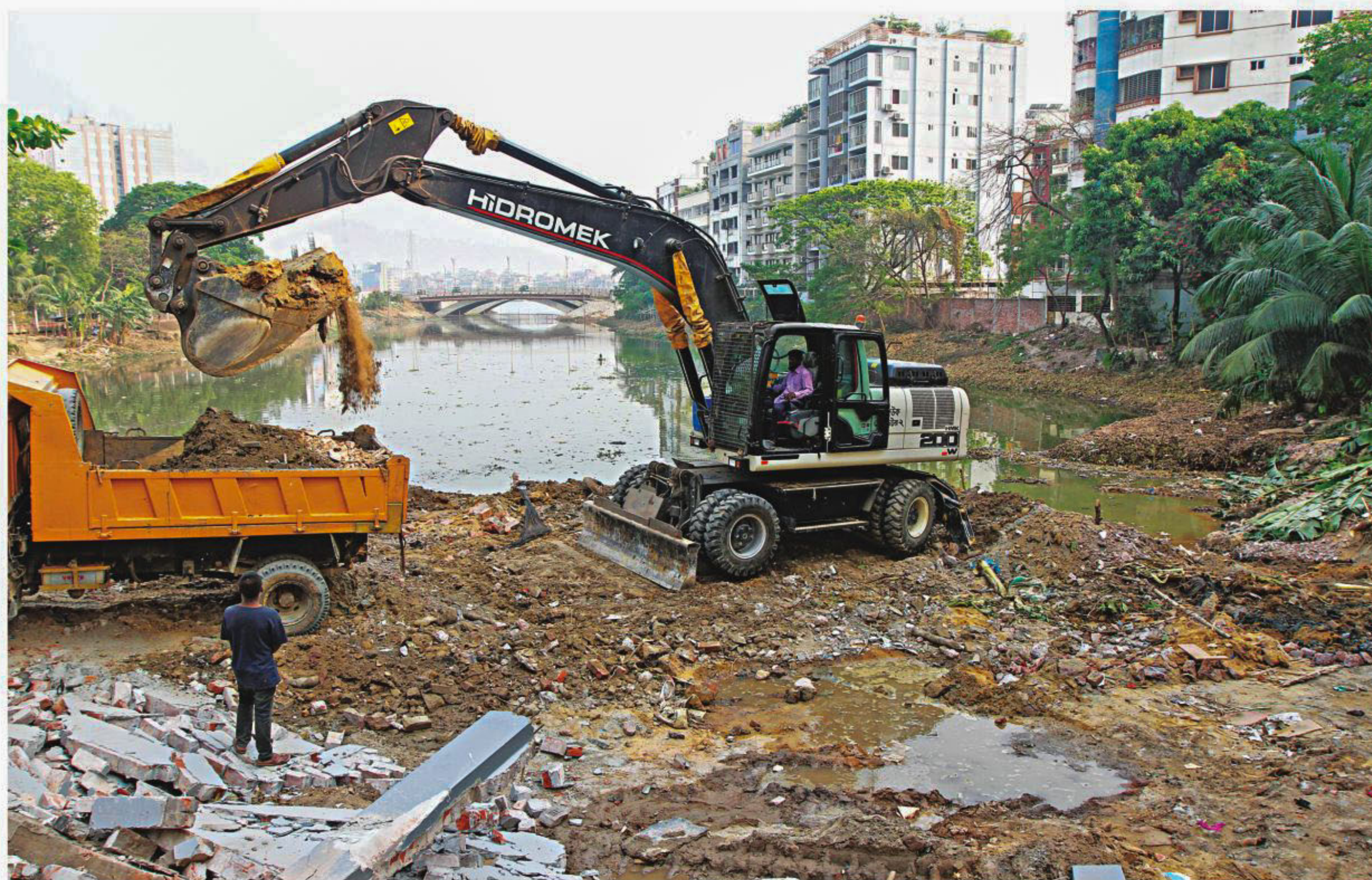
A claimant of a 10-katha piece of land in the Gulshan-Niketan Lake in the city's Gulshan had filled this portion of the water body near the Gulshan-Niketan bridge. The claimant had also planted some banana trees there. Rajdhani Unnayan Kartripakkha yesterday morning demolished the structures and removed some of the earth. The photo was taken near Niketon Gate yesterday.
