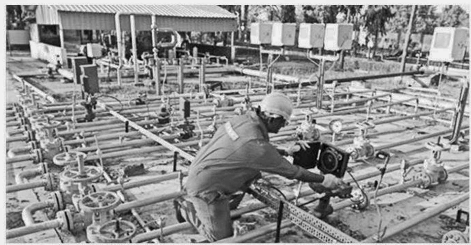
A technician works inside the Oil and Natural Gas Corp group gathering station on the outskirts of the western Indian city of Ahmedabad.
