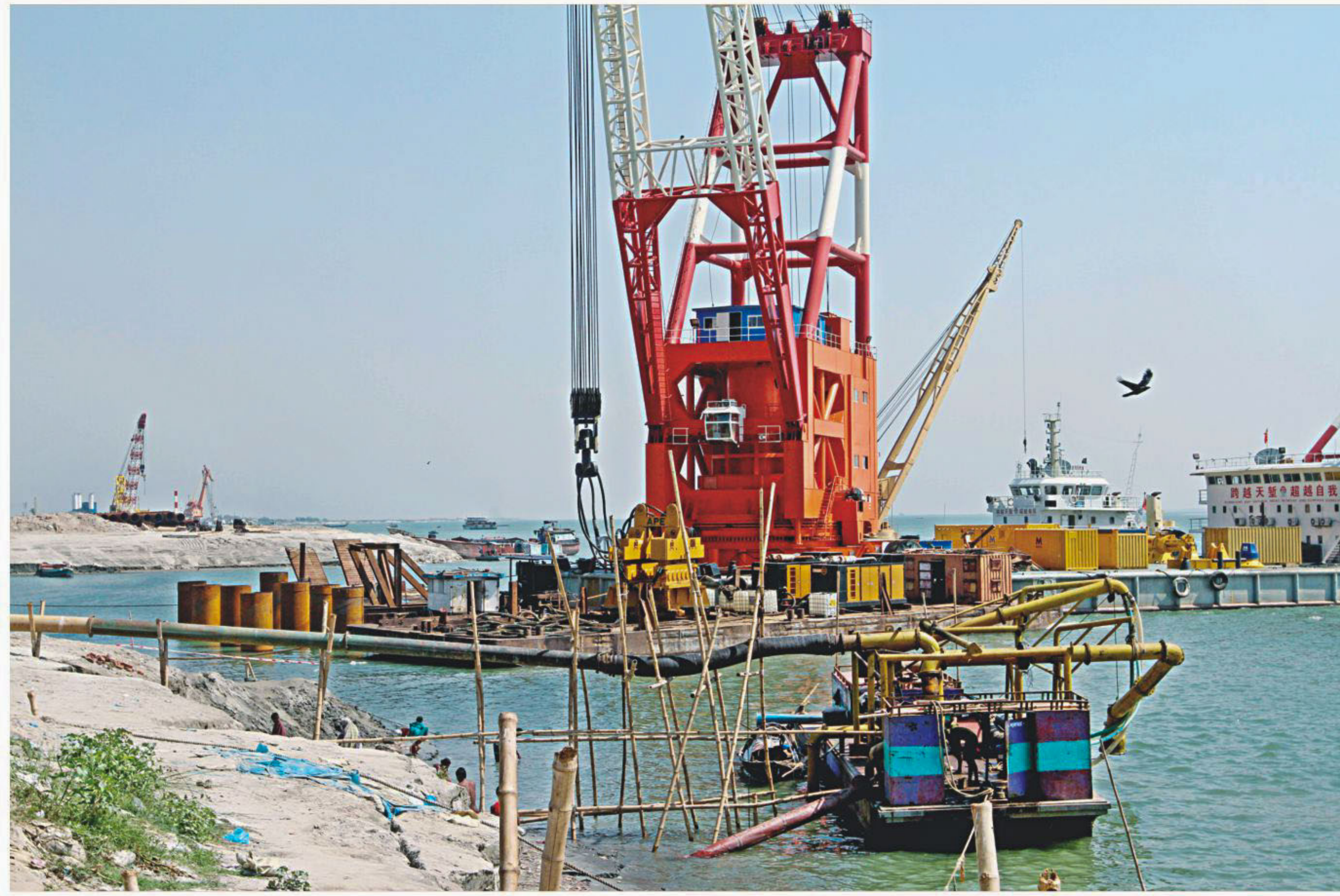
Construction of Padma Multipurpose Bridge going on in full swing, with 16 pile pipes for the second pillar already driven into the river bed at Mawa end. The much-awaited bridge connecting Dhaka with south-western districts is scheduled to open in 2018. The photo was taken on Tuesday. PHOTO: ANISUR RAHMAN
