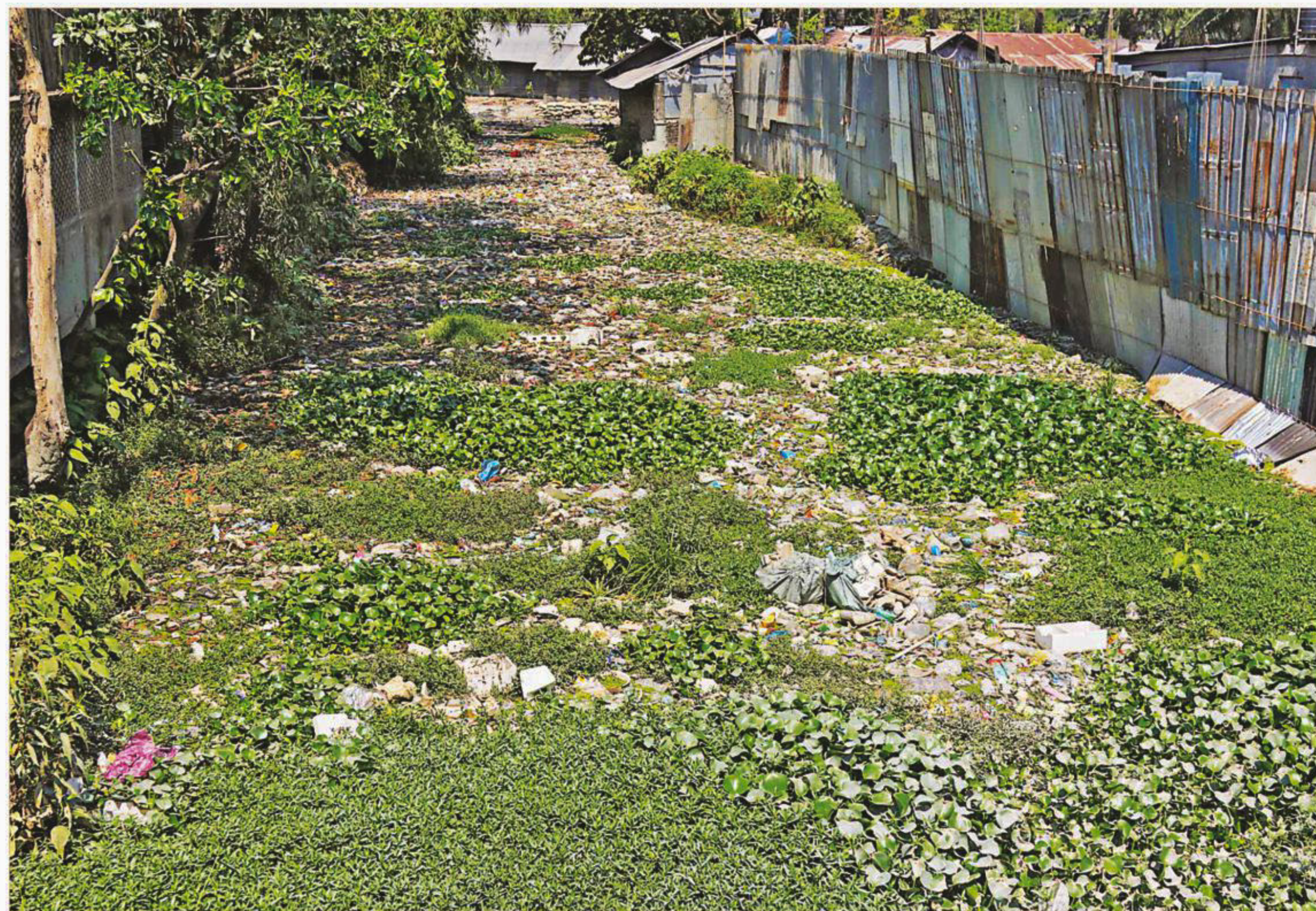
Mariam Khal, a drainage canal in Pathargata of Chittagong city, has been choked with garbage and water-hyacinths and narrowed down through encroachment on both banks, resulting in waterlogging in the neighbourhood even after light rains. The photo was taken yesterday.
