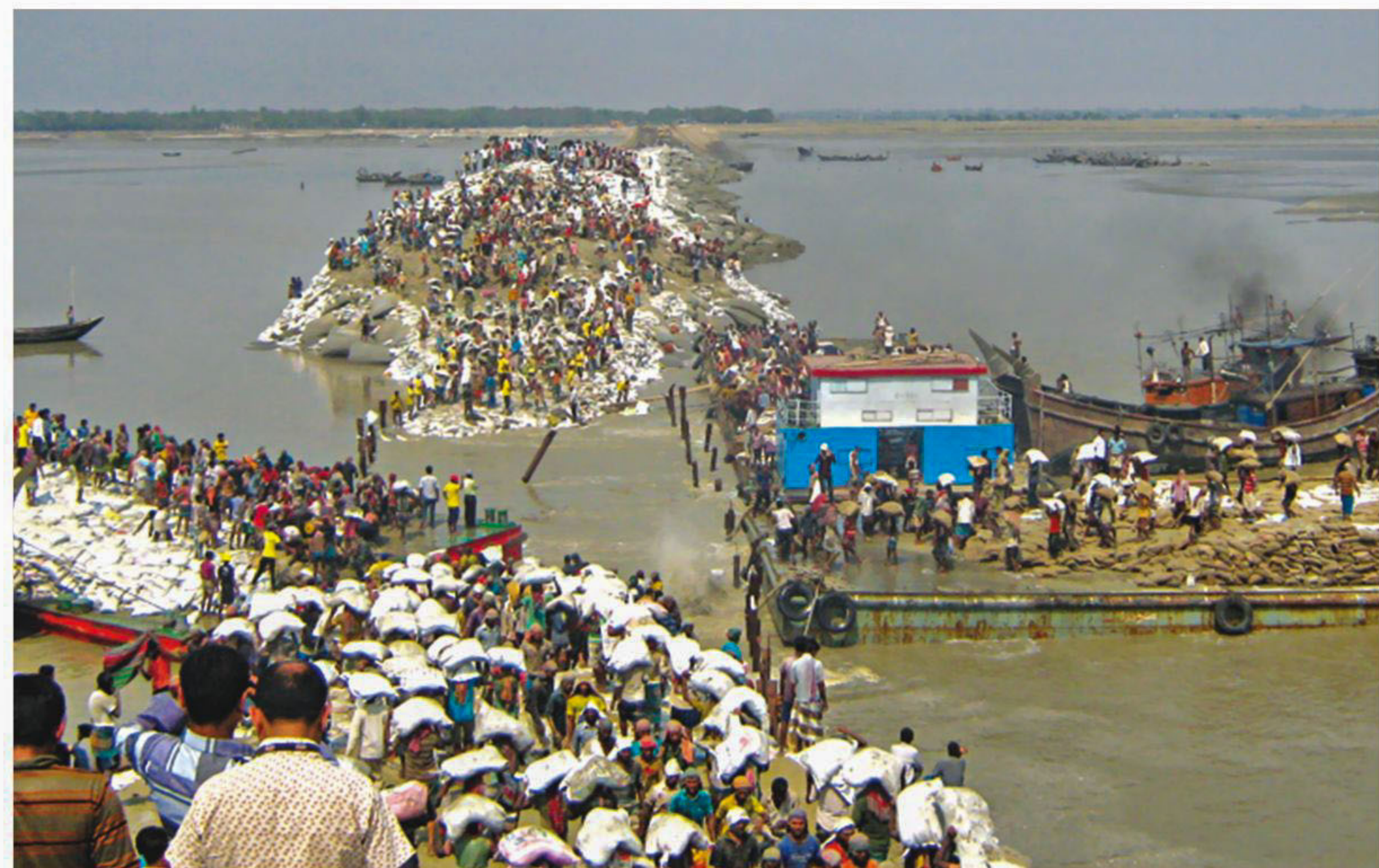
The Musapur closure at Companiganj in Noakhali washed away by heavy current of the river Chhoto Feni, three hours after it was opened on Saturday.
