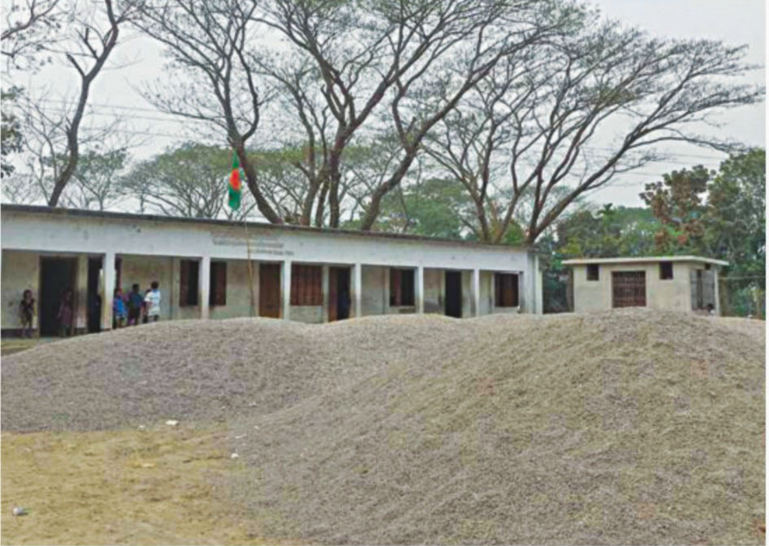
Construction materials occupy the ground of Narayanpur Government Primary School in Ishwarganj upazila of Mymensingh district, disturbing classes and extra-curricular activities of the kids and posing health hazard for the learners and teachers.
