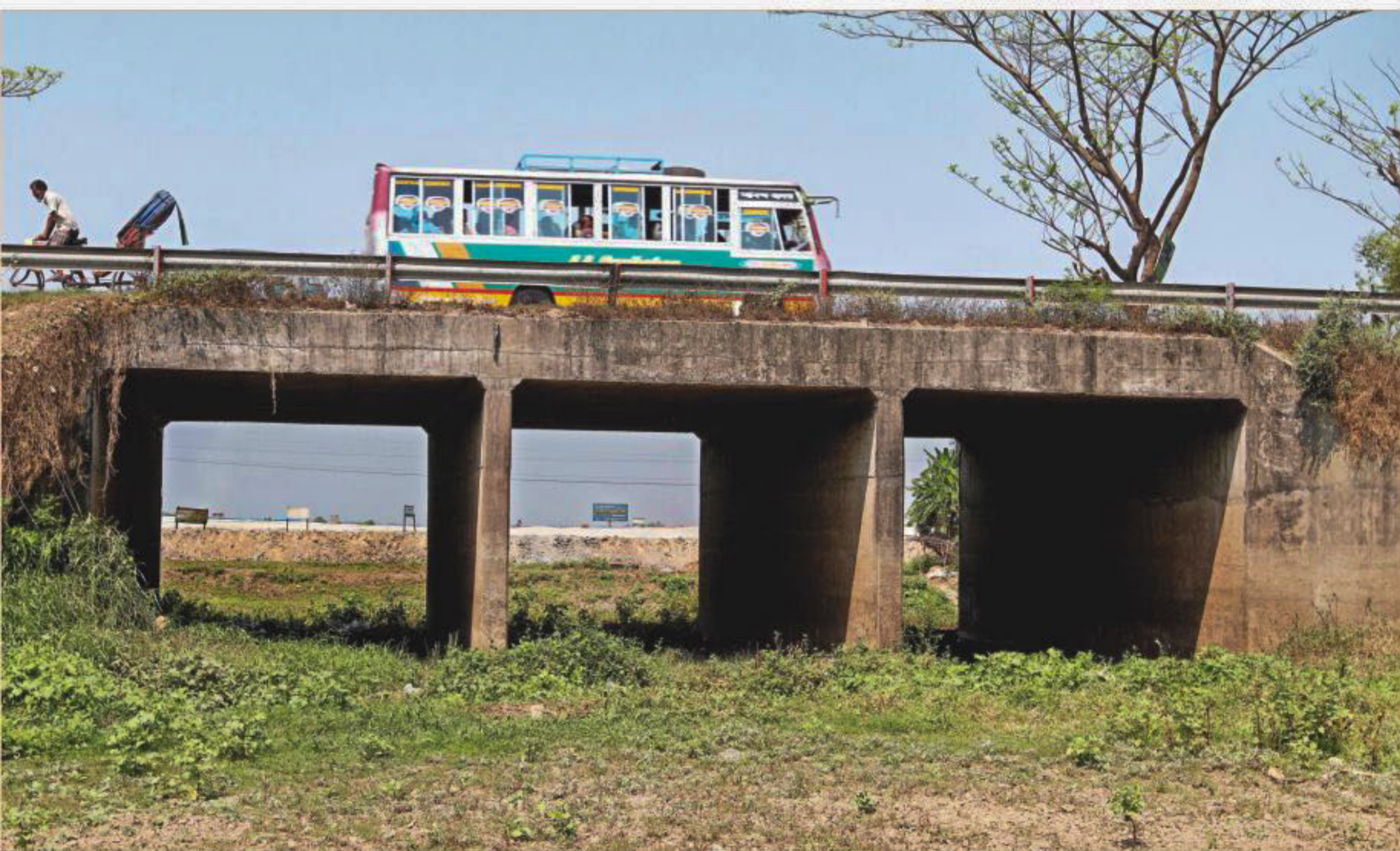
This culvert has virtually lost its use because of rapid land development on both sides replacing vast wetlands along the Dhaka-Mawa Highway, just outside the capital. The photo was taken yesterday in Keain of Munshiganj that testifies to how unplanned urbanisation is wiping out the swamps, which are an integral part to maintain the environmental balance.
