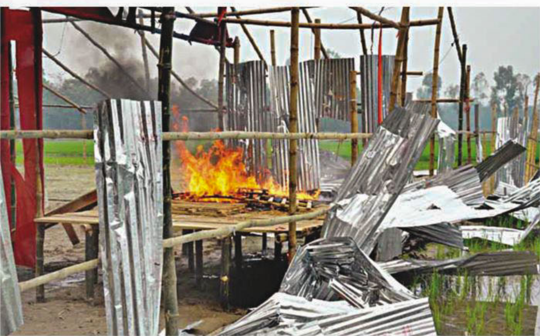
The district administration destroys this structure along with another one at Dholbhangra Bazar in Palashbari upazila under Gaibandha district yesterday as the spots were being used for holding obscene dance and gambling in the name of jatra (open stage drama).
