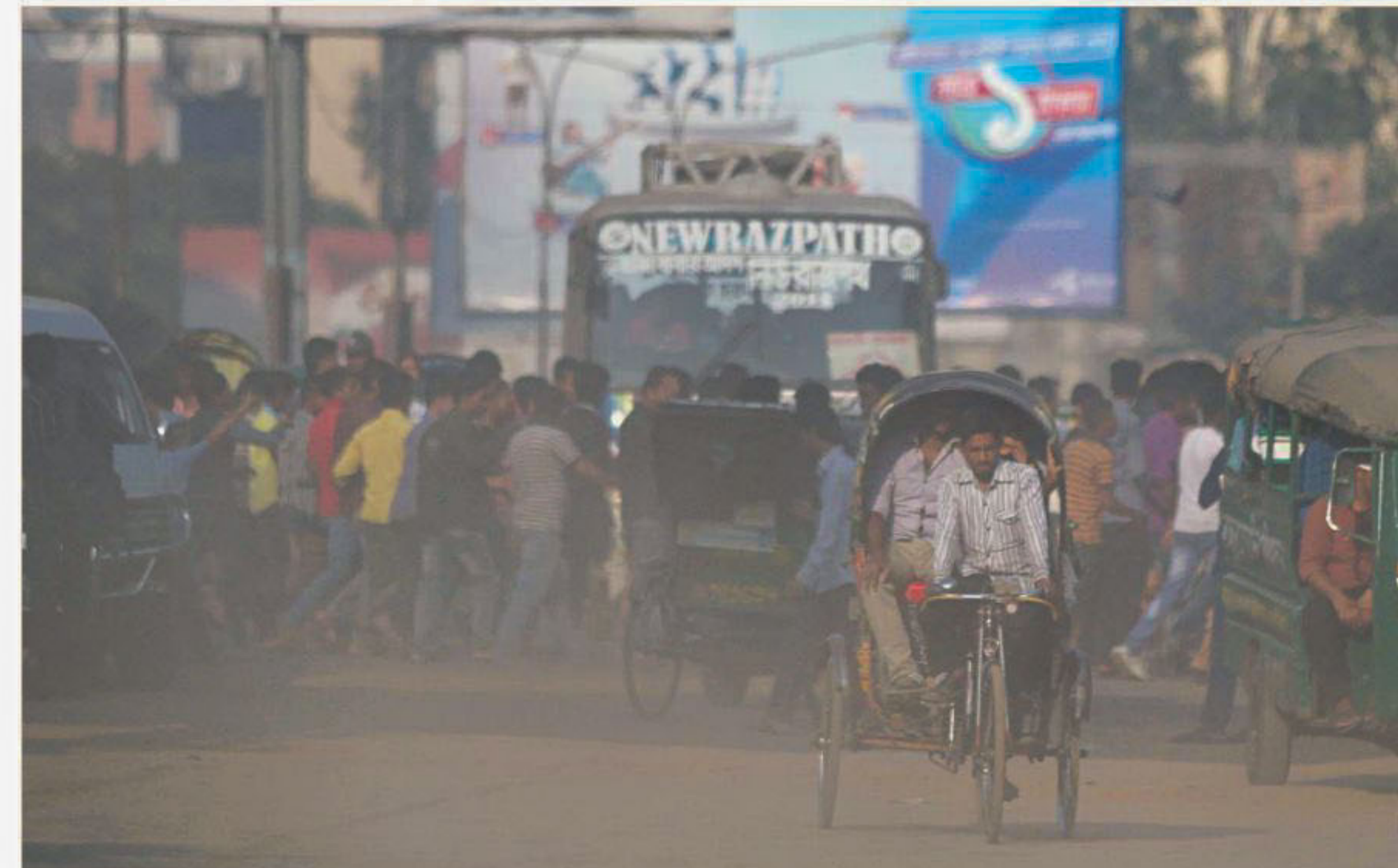
A leading cause for respiratory problems, dust clouds, aided by the dry winter weather, swirl up from earth being dug up by Chittagong Water Supply and Sewerage Authority for the installation of pipes on the Ispahani intersection in Chittagong city around noon yesterday.
