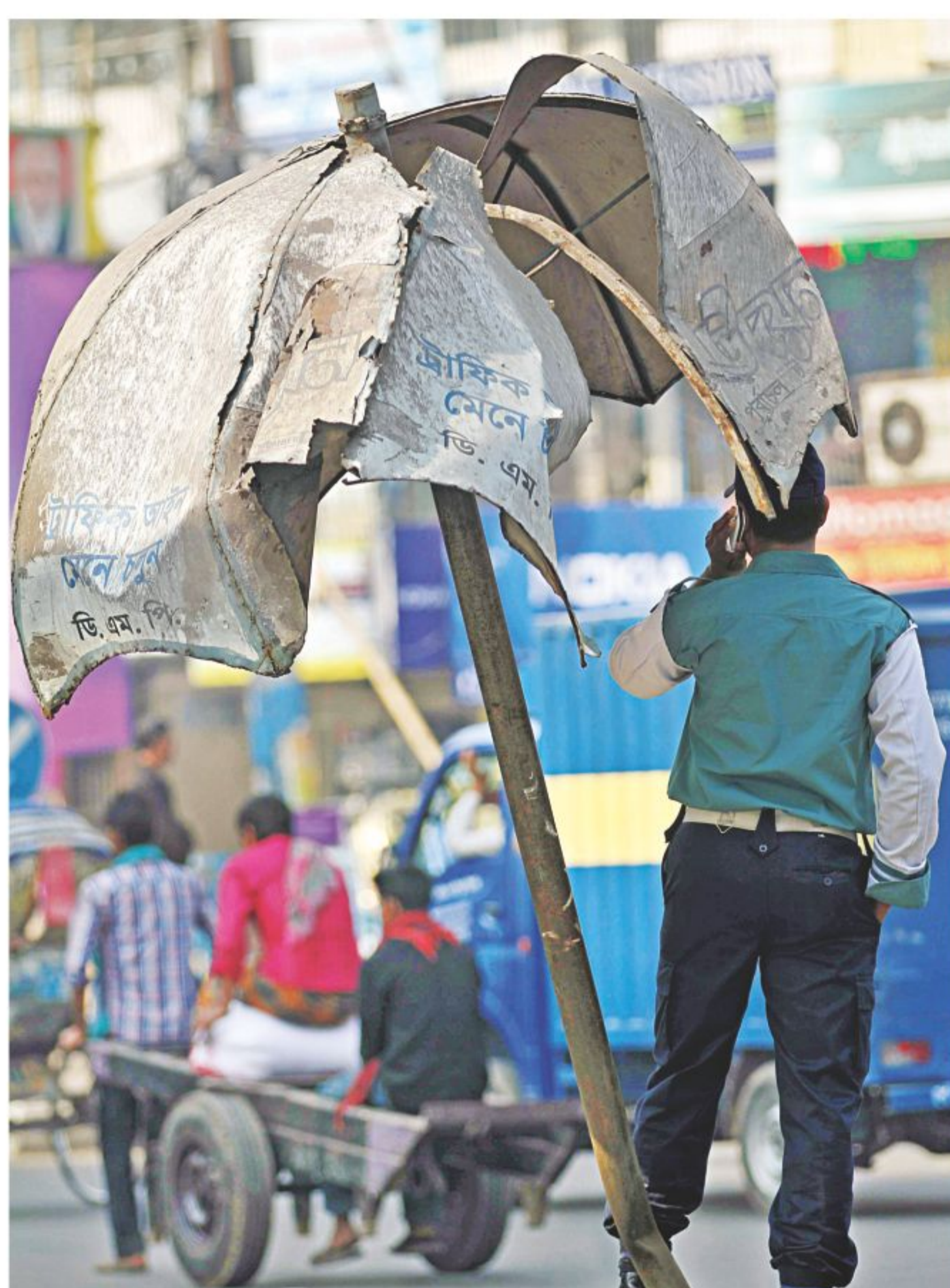
This recently taken photo shows a traffic police standing under what used to be a shade before being bent and mangled by a vehicle over a year ago at the capital's Fakirapool intersection.
