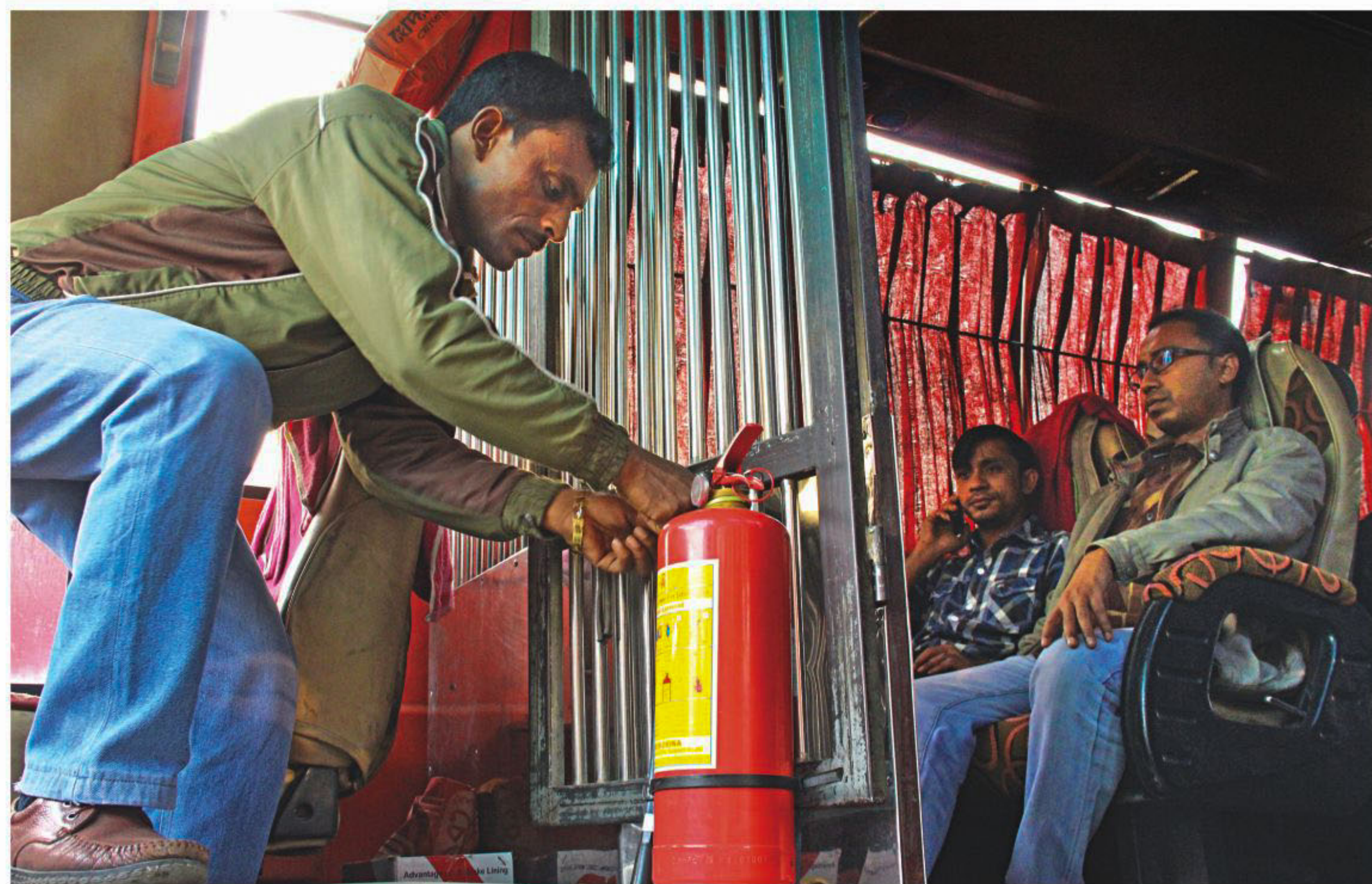
A fire extinguisher being installed inside a bus at Mohakhali Bus Terminal yesterday. This is a precaution the bus owners are taking with incidents of petrol bomb attacks on buses on the rise since the nationwide indefinite blockade was enforced earlier this month.
