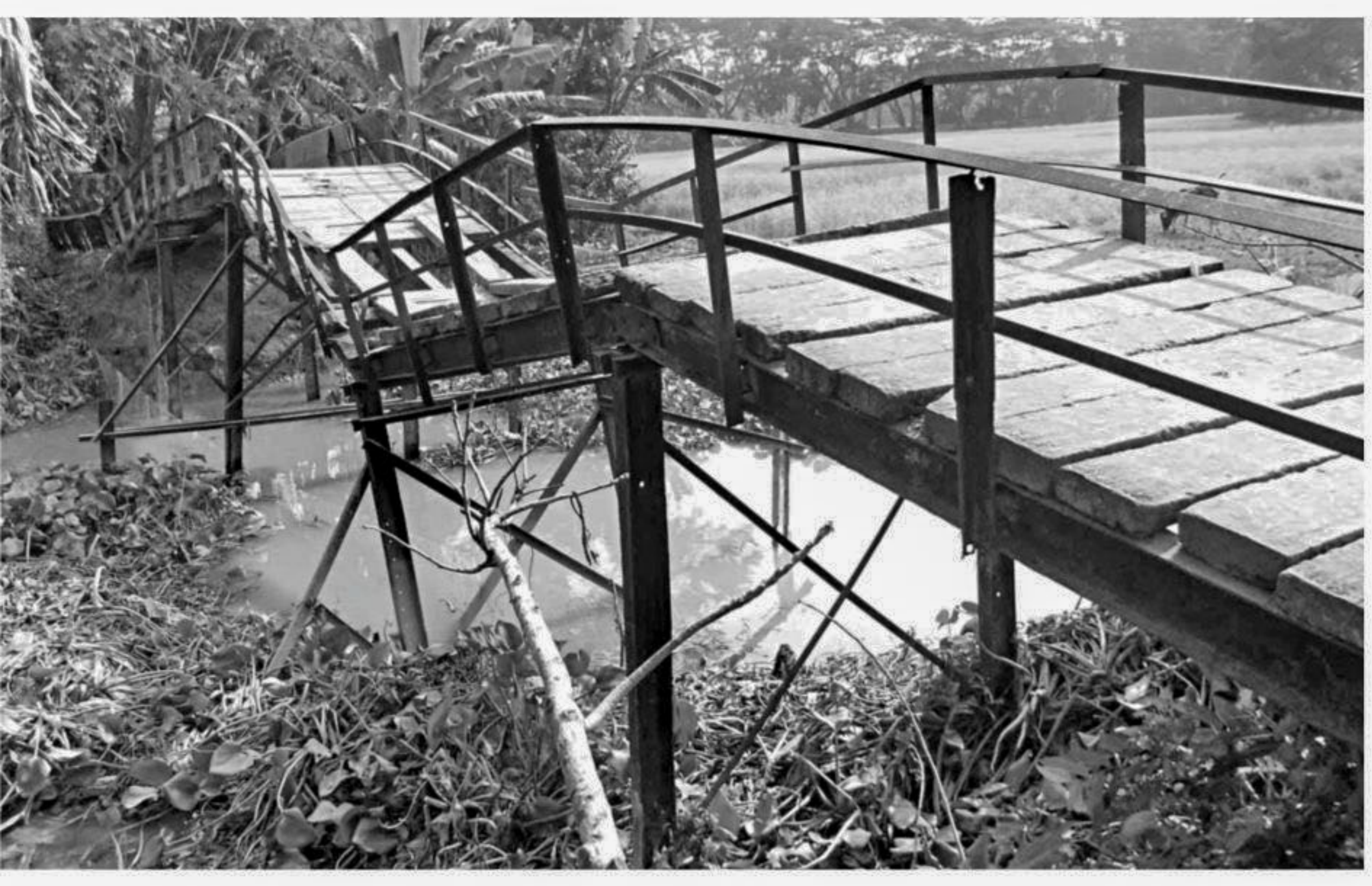
A large number of people have to use this awfully risky bridge over Kismotpur canal on Shingbari-Sultanabad road in Mirzaganj upazila under Patuakhali district as the authorities concerned did not repair the structure five years after its partial collapse.
