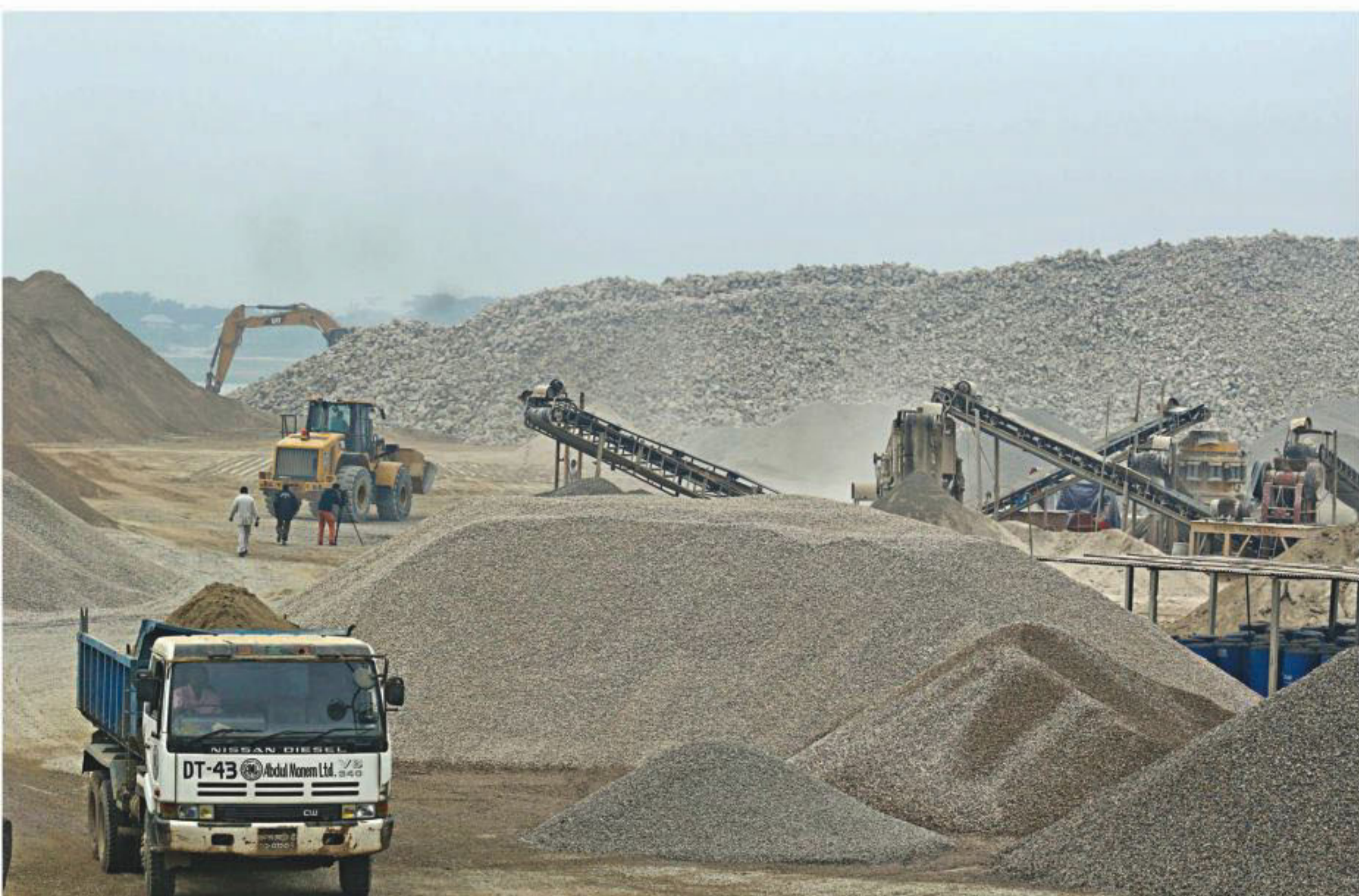
Trucks and earth-moving equipment preparing the materials for the Padma bridge at the construction site. The photo was taken recently.
