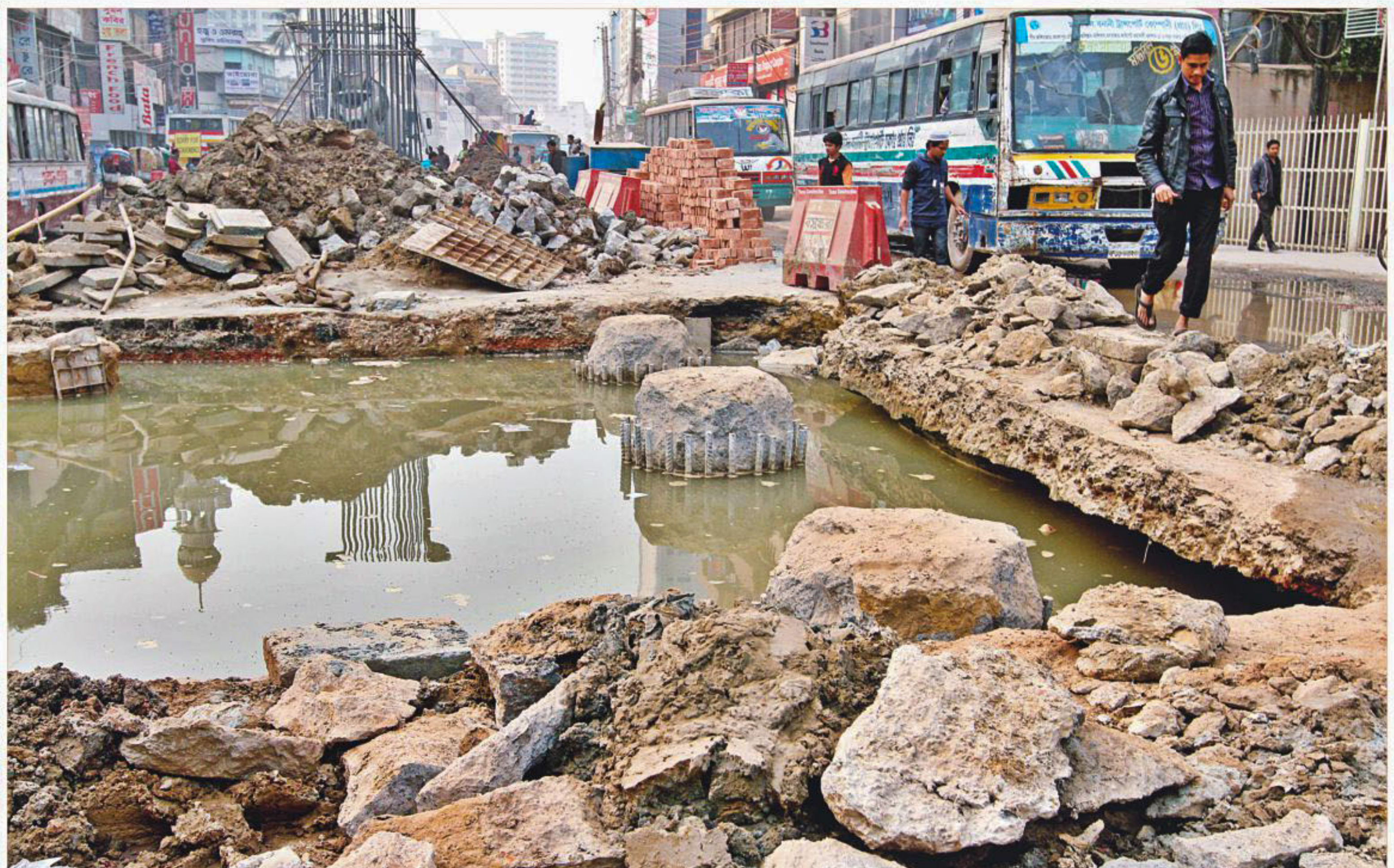
Water leaking out from ruptured sewerage pipes has created a new danger in the unguarded construction site of Moghbazar-Mouchak flyover in the capital, by washing away earth from underneath the narrow strip of the road left available for vehicular traffic. The photo was taken yesterday, in front of the Mouchak market.
