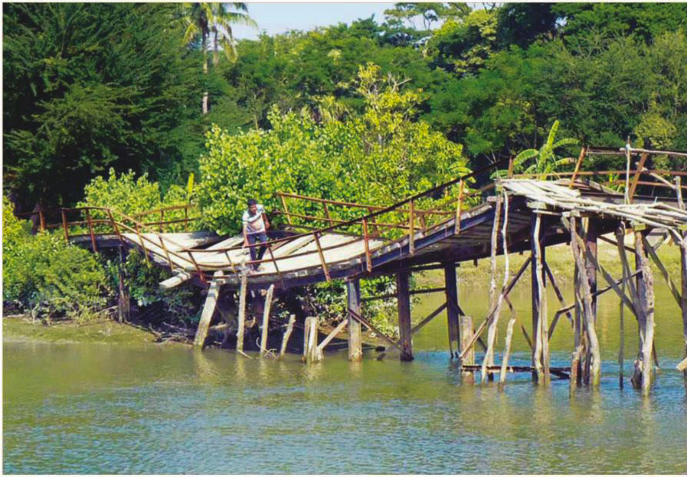
Unbelievable as it may seem, this rickety bridge over the Thonju Para canal of Kuakata is being used every day by hundreds of locals, including children of four schools, braving the risk of an accident. The photo was taken yesterday.
