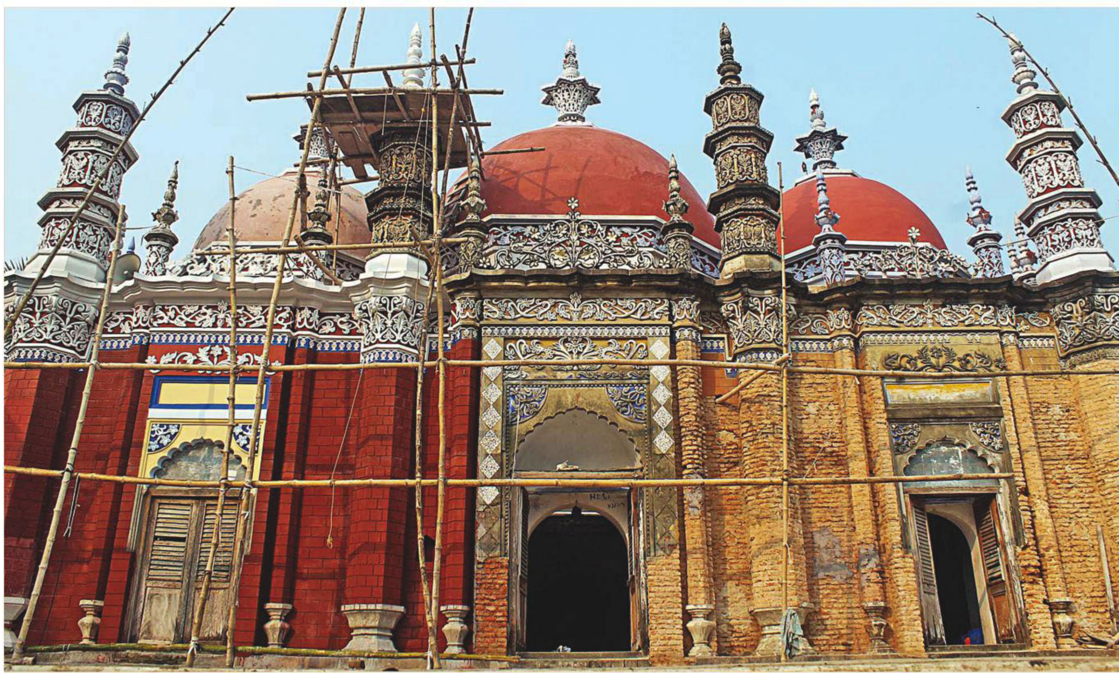
ABOLITION IN NAME OF RESTORATION Renovation works on Karapur Mian Bari Mosque, believed to be over 300 years old and situated in North Karapur village under Barisal sadar upazila, by self-proclaimed descendants of the mosque's founders have resulted in an alteration of the original colour and facade. The locals, however, are for keeping the mosque in its original form. The photo was taken recently. PHOTO: ARIFUR RAHMAN
