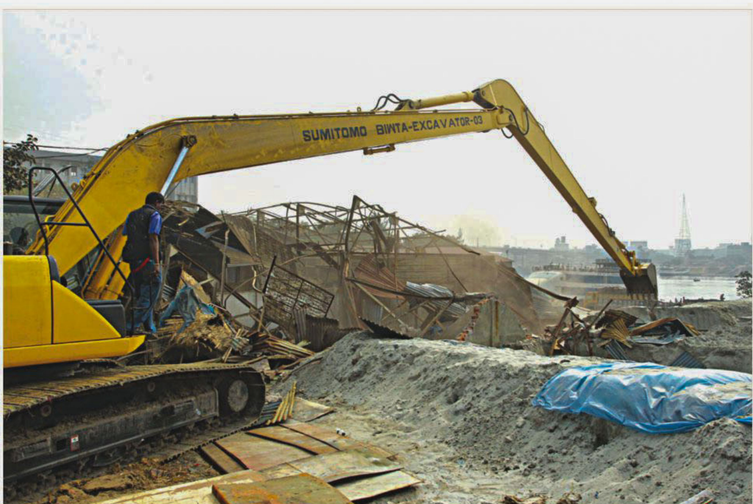
Bangladesh Inland Water Transport Authority yesterday demolishes illegal structures which had encroached on the banks of the Buriganga river in Postogola Shashan Ghat area in the capital.
