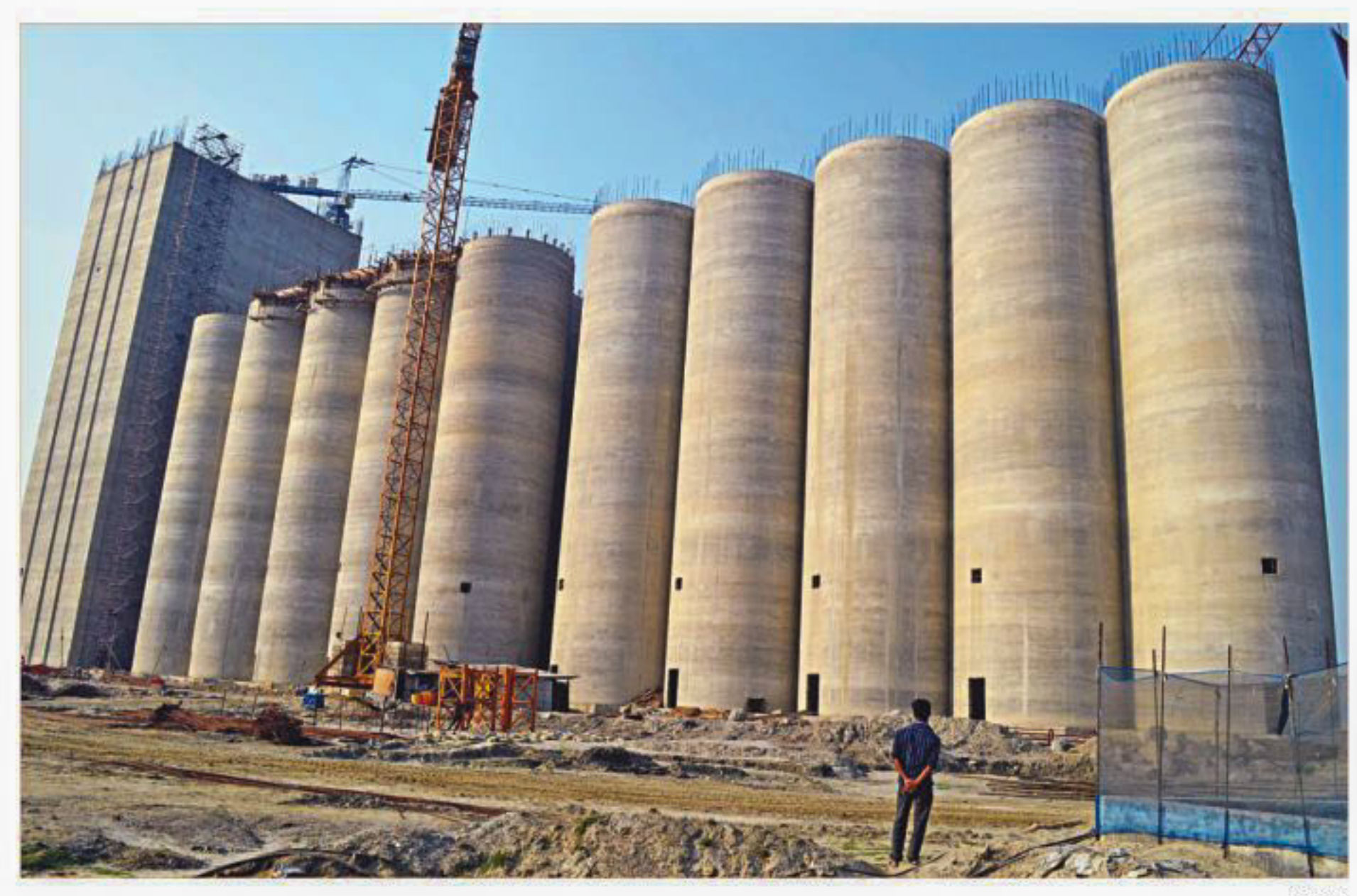
A man looks at the 50,000-tonne grain silo under construction in Joymony village on the bank of the Pashur River in Mongla. Almost 65 percent work is complete.
