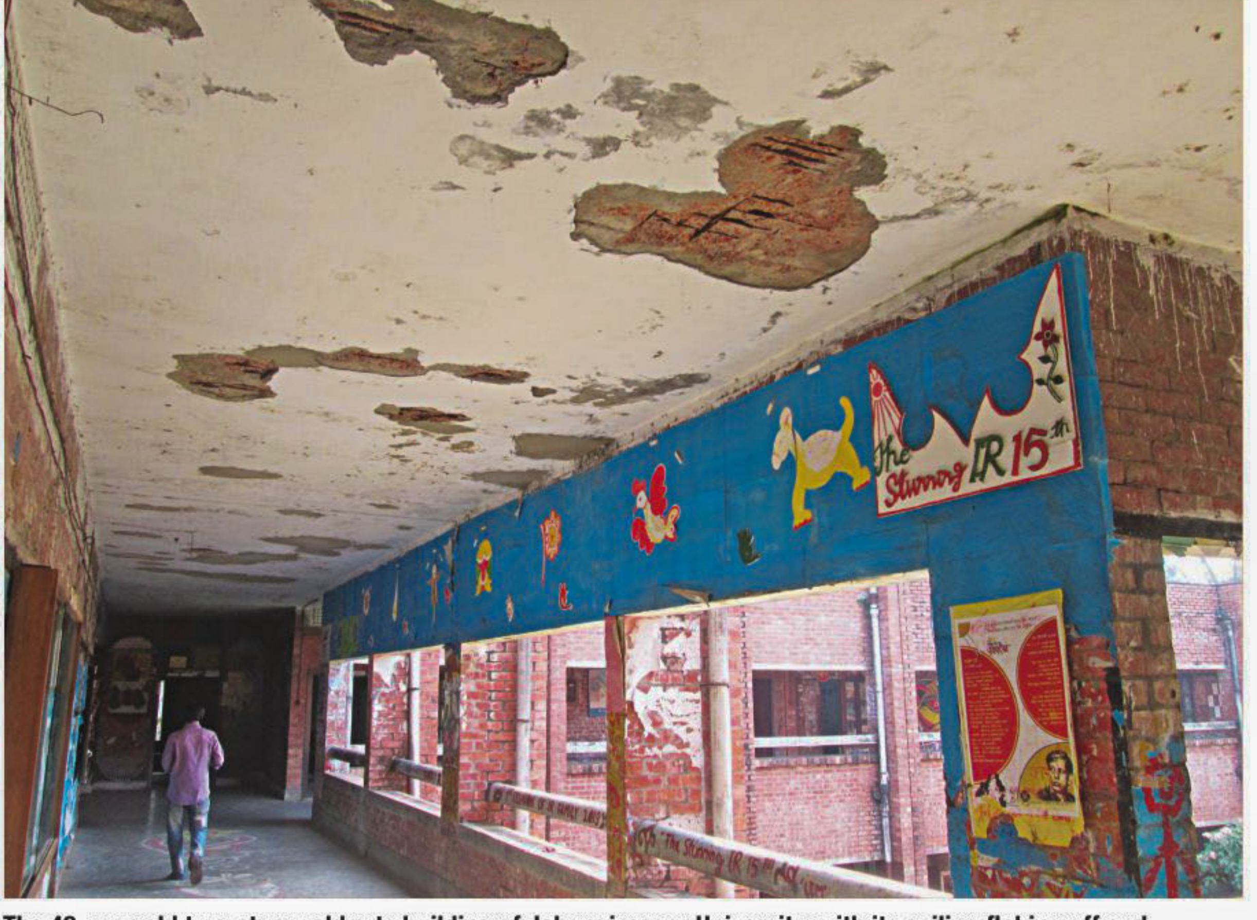
The 42-year-old two-storey old arts building of Jahangirnagar University, with its ceiling flaking off and developing cracks, needs urgent repair works to prevent any sort of disaster. The photo, taken recently, portrays the first floor of the building which houses the drama and dramatics department. PHOTO: STAR
