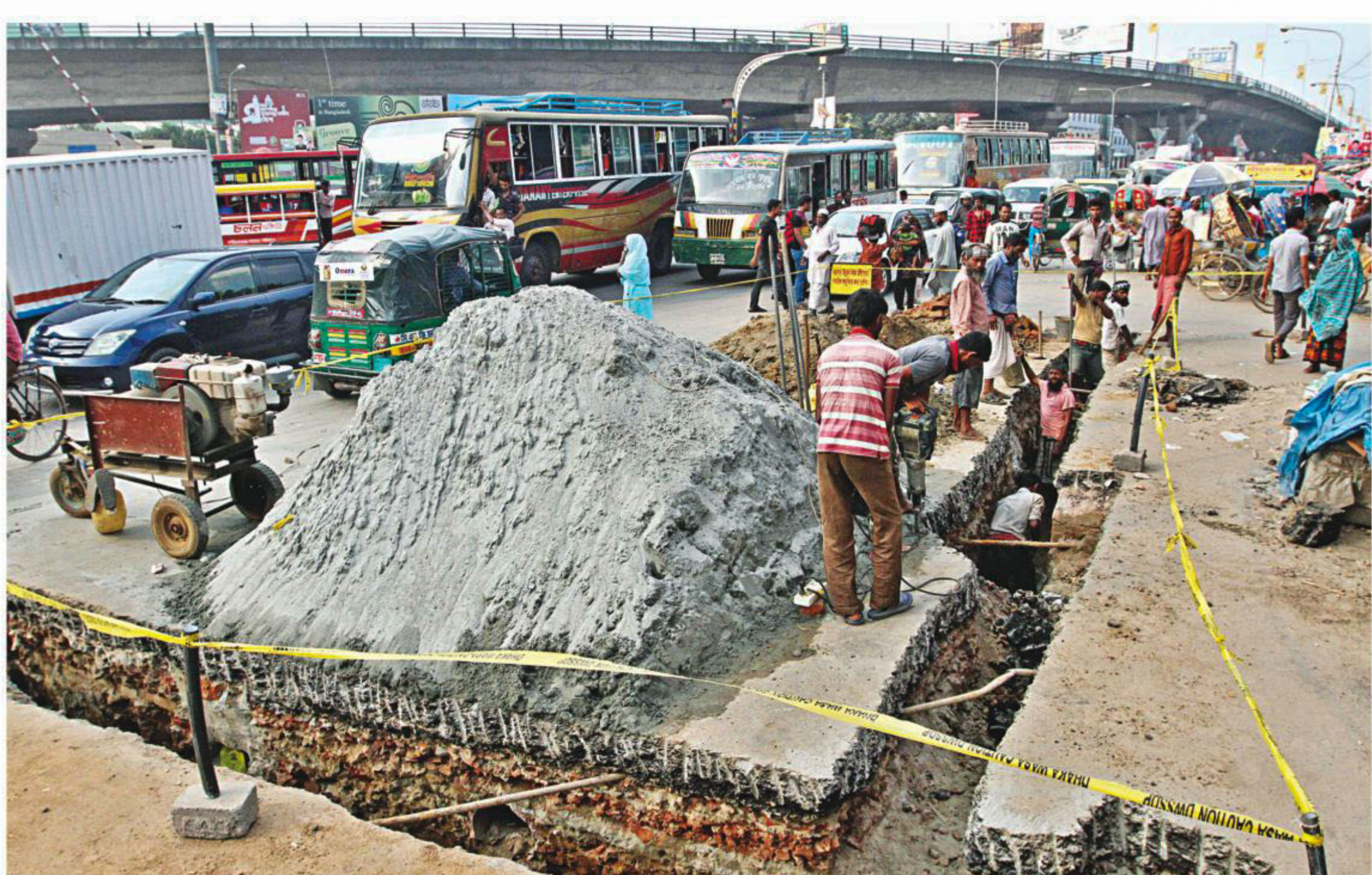
Sand has been piled up while the road, some distance before the Directorate General of Health Services in the capital's Mohakhali, dug up in a span of four days by Dhaka Water Supply and Sewerage Authority to carry out development works, causing traffic congestion due to the narrowing down of the road. The photo was taken on Friday.
