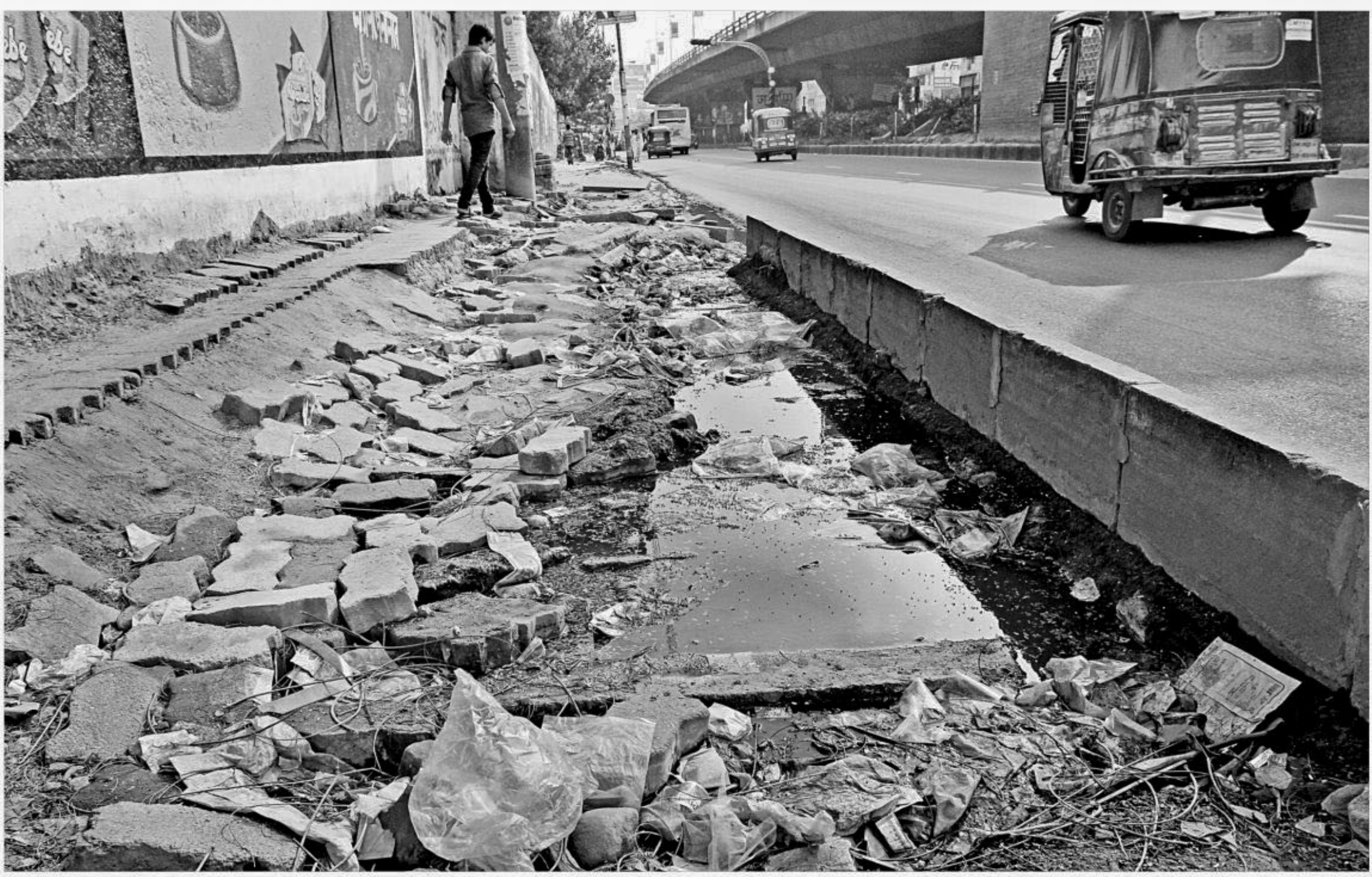
This footpath situated some metres before a left turn, which leads to Gulshan 1, while approaching from Chairmanbari in the capital has been in this state for around four months, apparently with the authorities concerned turning a blind eye. The photo was taken yesterday.
