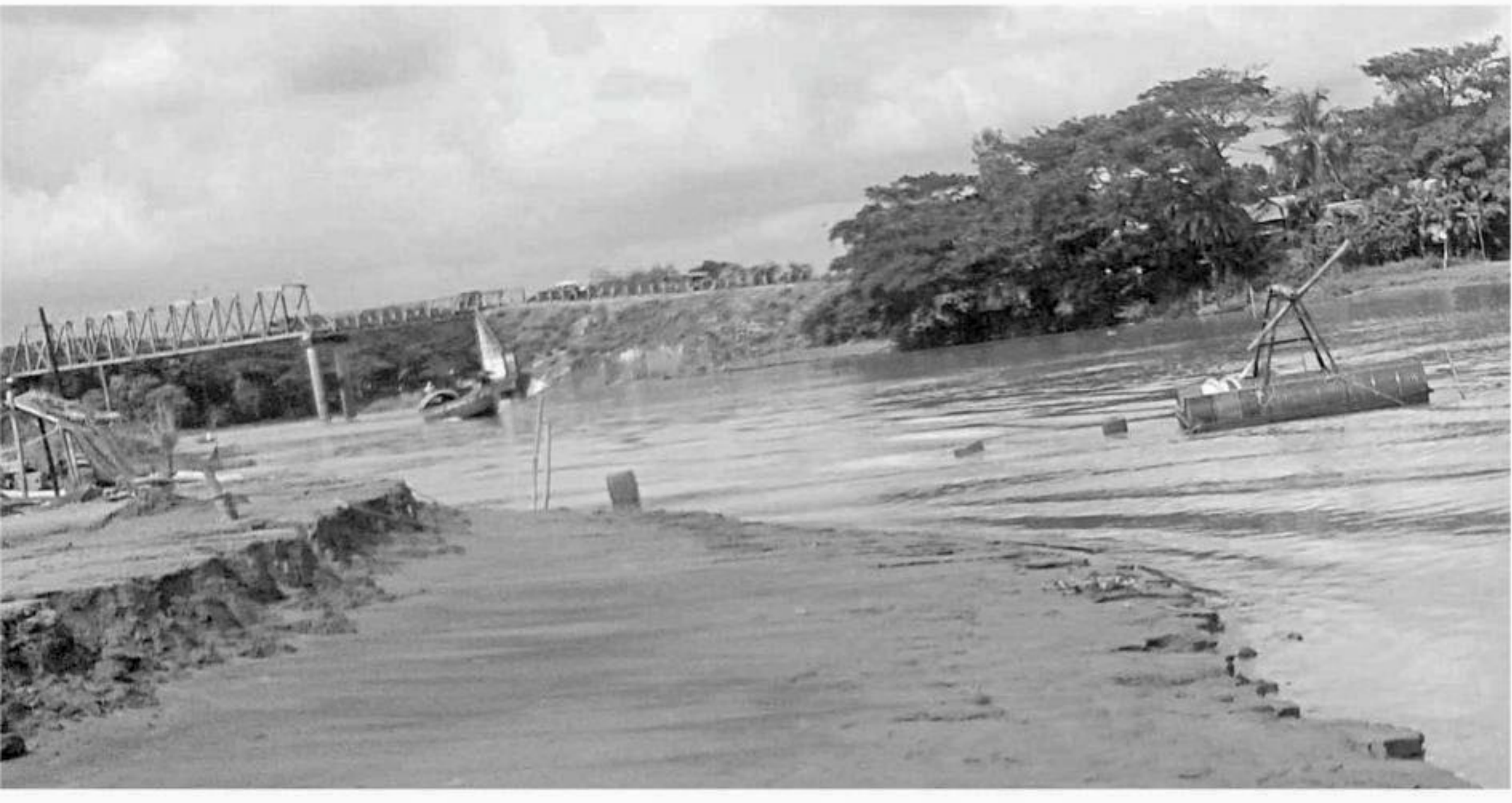
Massive sand lifting with dredgers from Taltali-Gouraganj canal near Kunderbazar bridge on Munshiganj-Sirajdikhan-Dhaka road in Tongbari upazila under Munshiganj district poses threat to the important bridge as well as nearby farmlands. Owner of a proposed chemical industry has continued the mindless act to fill up the bank of the government-owned water body.
