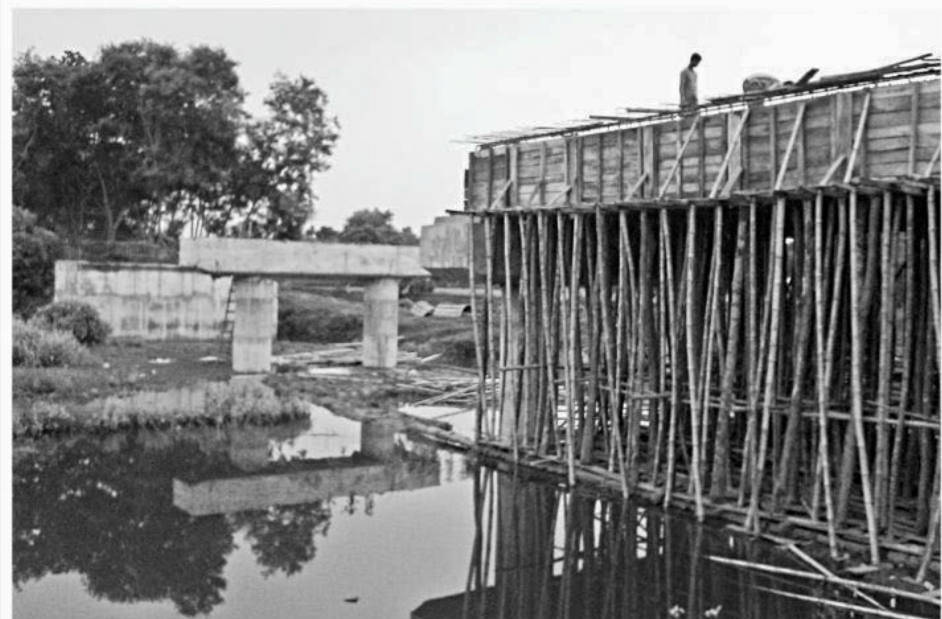
Construction work of Sitarampur bridge on Narail-Jessore road in Narail district has remained virtually stalled allegedly due to non-allocation of required fund, much to the frustration of thousands of commuters who travel amid risk through a temporary bridge on a diversion road.
