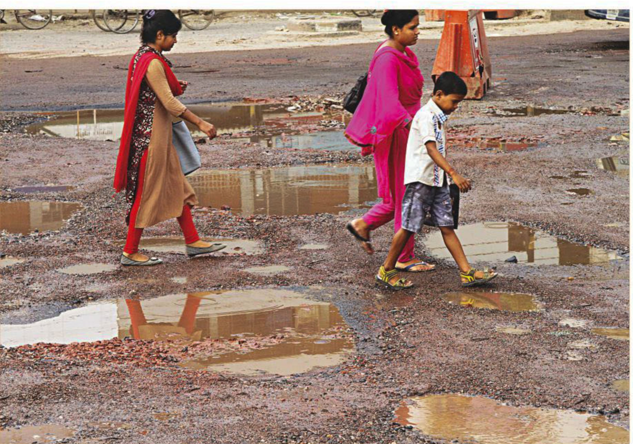
The same scenario was depicted in a photo published in The Daily Star a few months ago but the urgency for repairing the road, situated north of Malibagh Rail Crossing, failed to draw the attention of the authorities concerned. The new photo was taken yesterday.
