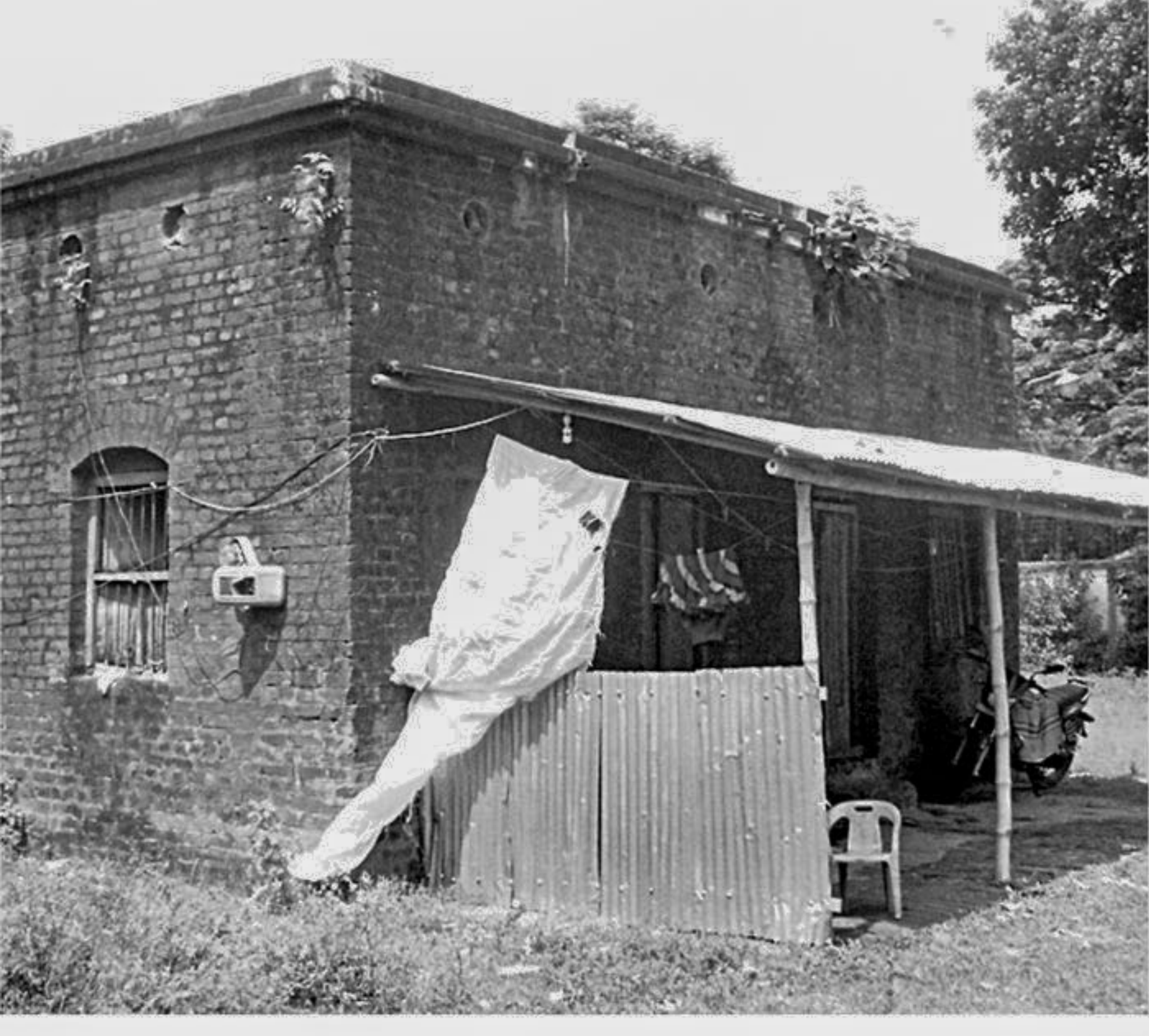
This decades-old building meant for staying of on-duty constables of Phulbari Police Station in Dinajpur district remains in an awful condition, posing risk of serious accident anytime.
