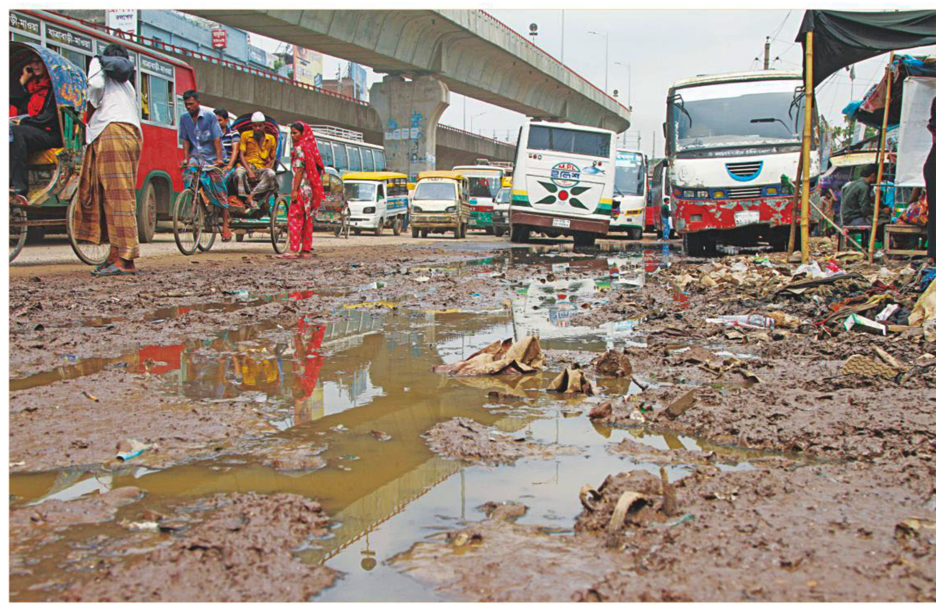
Sludge mixed with rainwater on the battered part near Jatrabari intersection is actually typical of the conditions of many Dhaka city streets. The results are perennial traffic chaos and frequent accidents. Such craters dot half-a-kilometre stretch of Jatrabari-Dholaipar road beside the Jatrabari ramp of Mayor Hanif flyover. The photo was taken yesterday.
