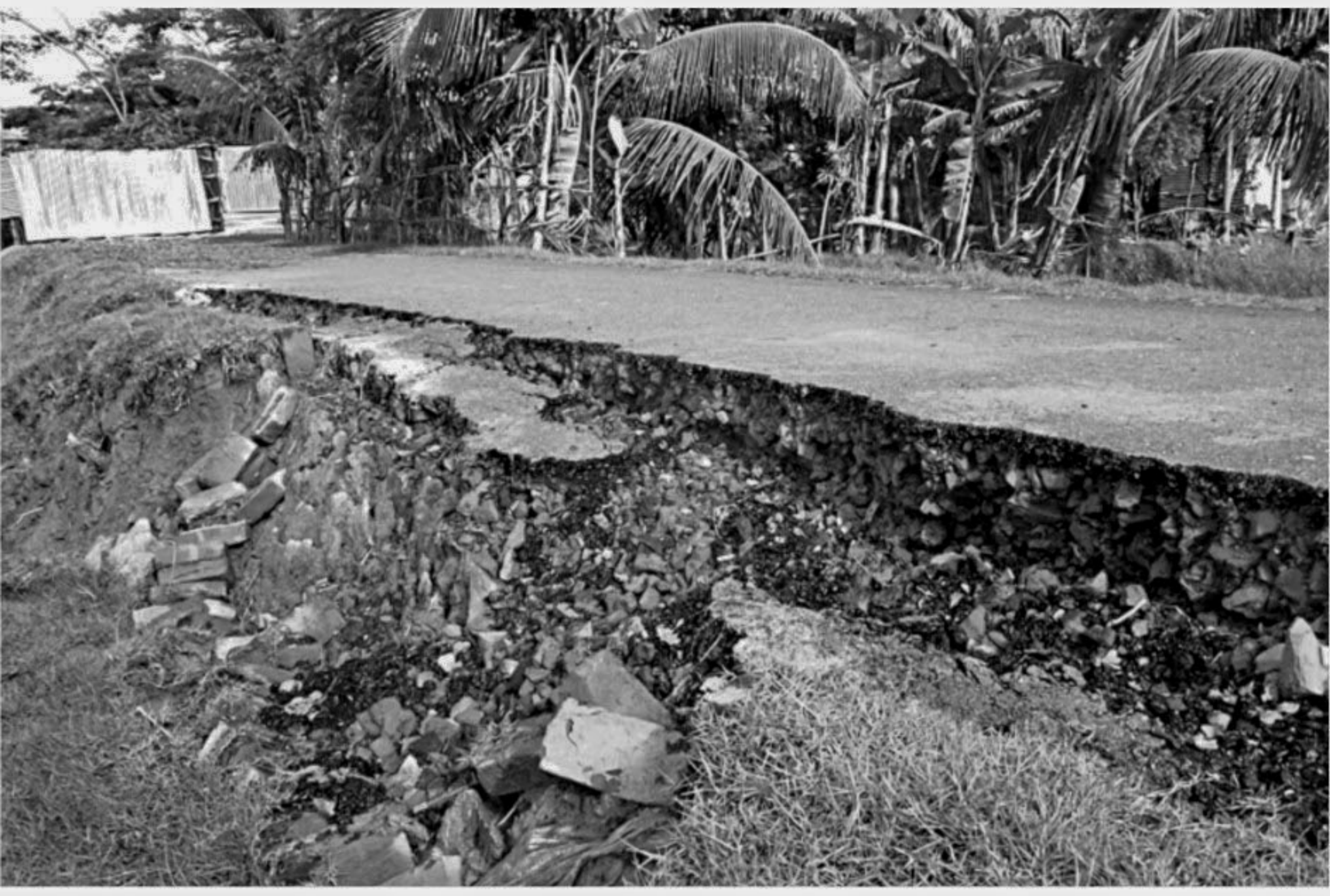
Around 975 metres metalled road, stretching from Kalapara Fire Service Office to Nachnapara Bashanti Mondol Government Primary School in the upazila of Patuakhali district, subsided at different points three months into its renovation.
