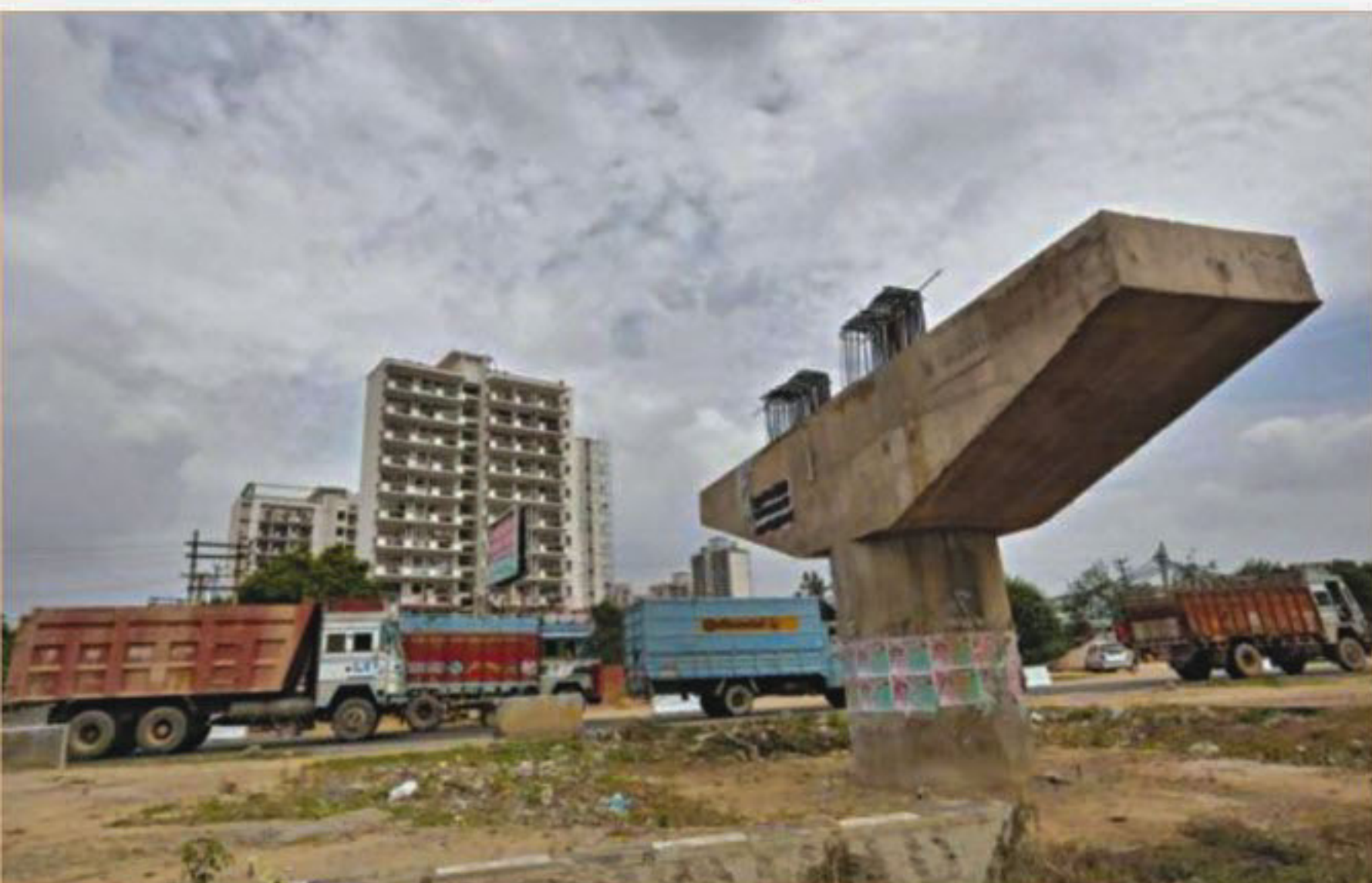
Vehicles travel past a Delhi-Jaipur national highway flyover under construction at Manesar in Haryana, India.
