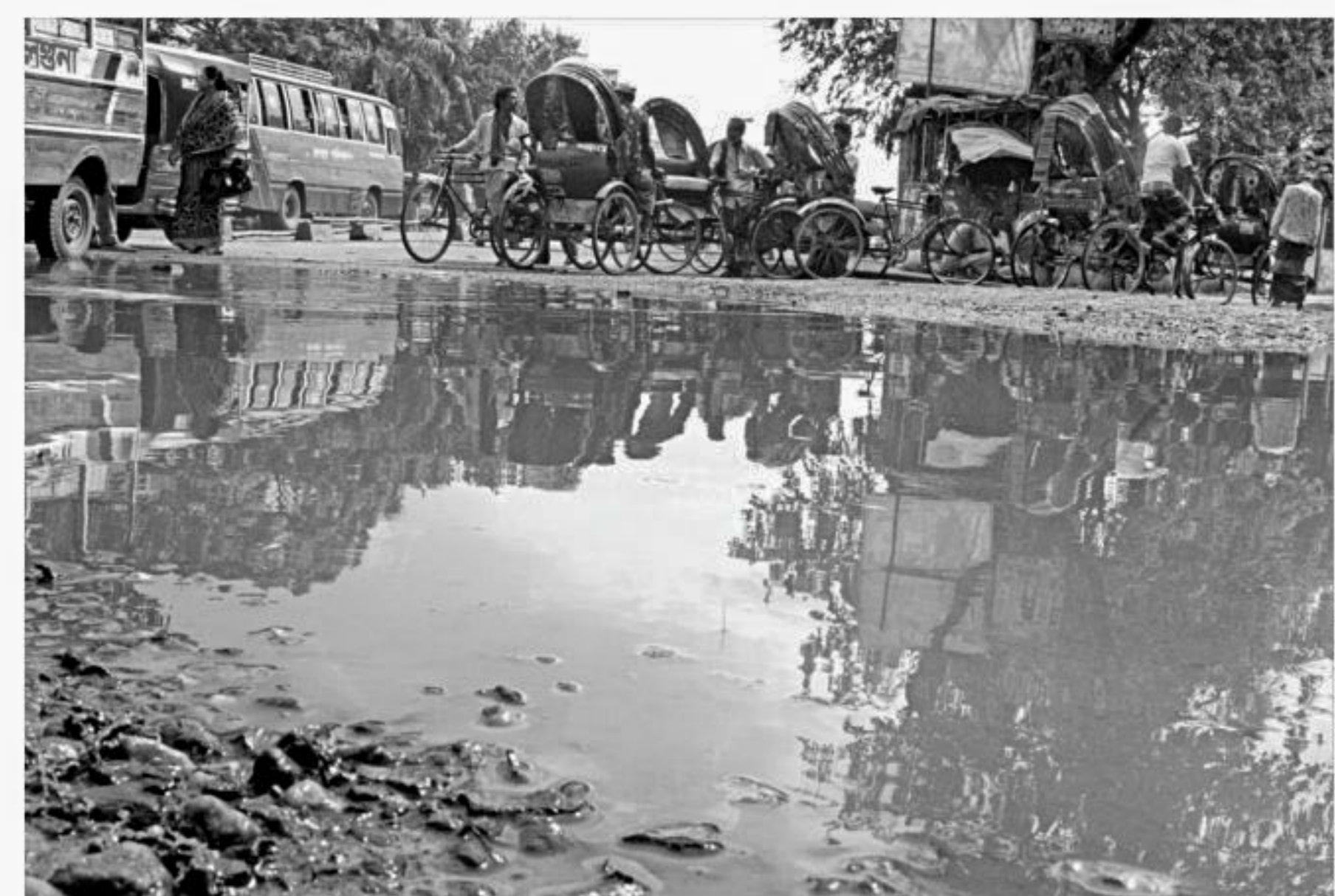
This pothole filled with water on the approach road north of Bangladesh-China Friendship Bridge makes vehicular movement difficult on the street. The road has been in this dismal state for quite a while with the authorities concerned turning a blind eye. The photo was taken on Tuesday in the capital's Postogola.
