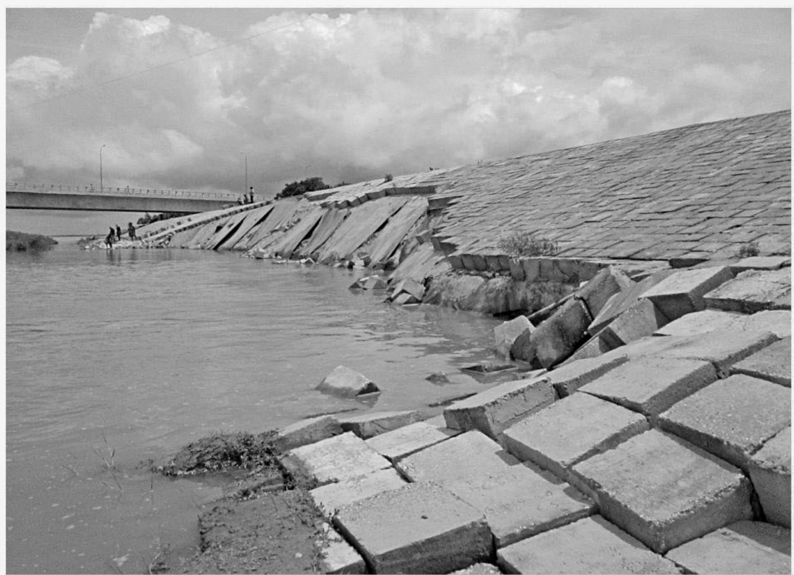
Around 100 metres of Teesta road bridge protection dyke over the Teesta River collapsed due to the onrush of water from upstream in Sadar upazila of Lalmonirhat yesterday.
