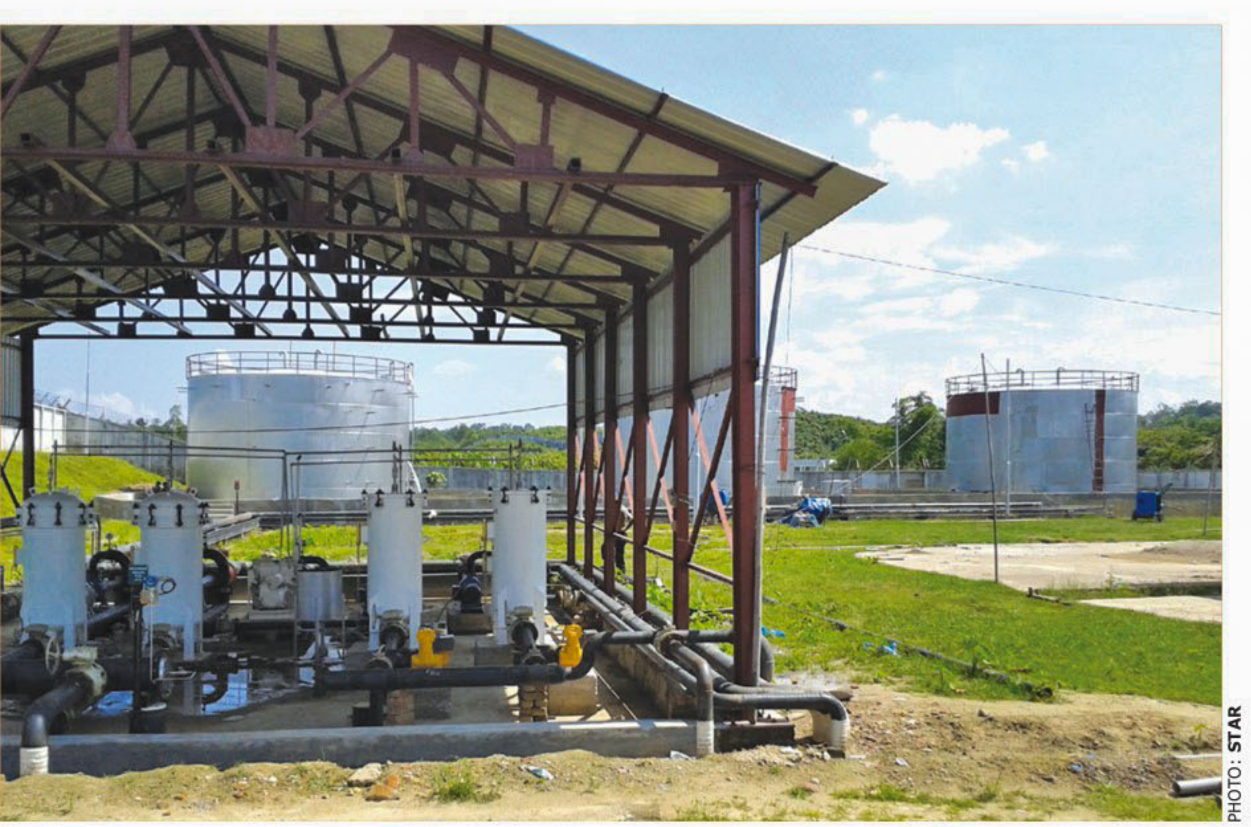
Three newly-built fuel storage tanks and other installations at Sylhet Osmani International Airport in Sylhet city. The airport had been lacking refuelling facilities for the last 16 years since it was declared international in 1998, and thus was unable to return international flights, which landed at the airport. The fuel station is expected to start operation in August.
