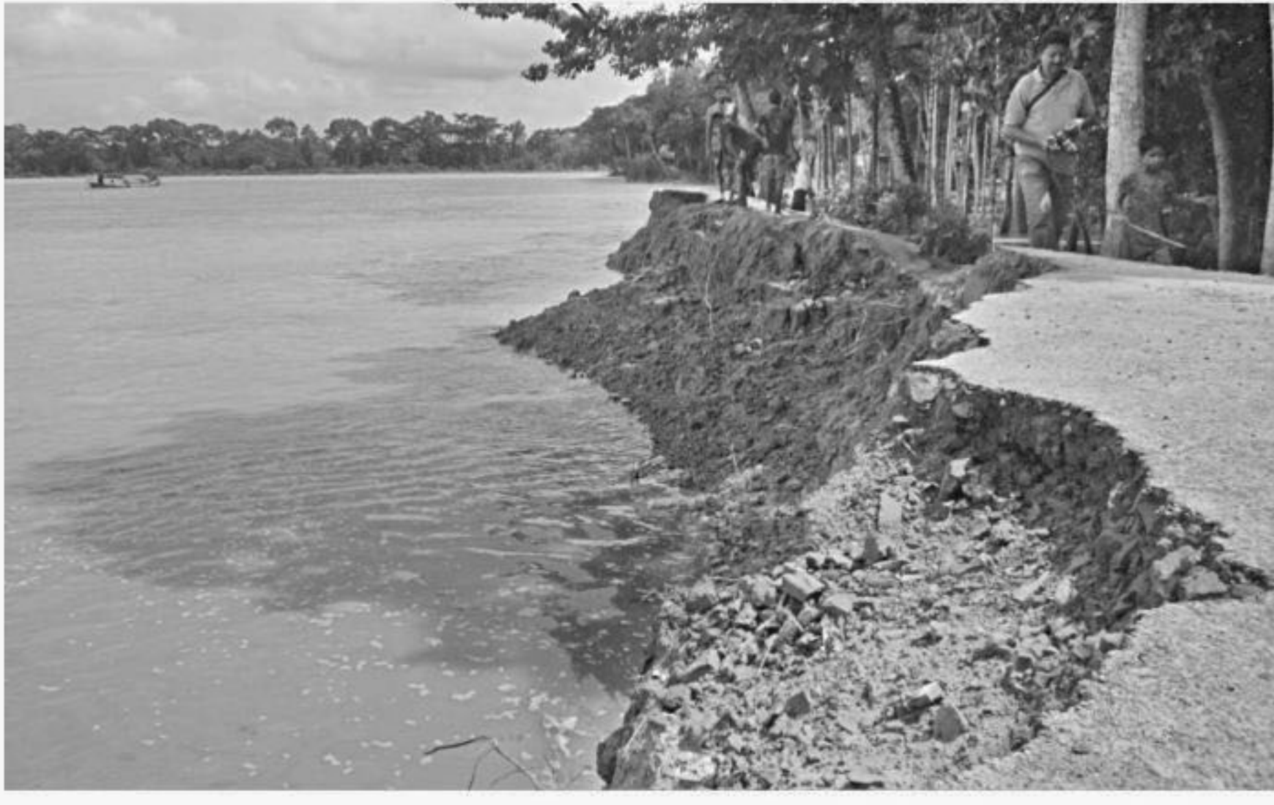
Over 300 dwelling houses at three villages under Patuakhali Sadar upazila have been inundated following collapse of a flood control dyke at Balaikathi point in the upazila
