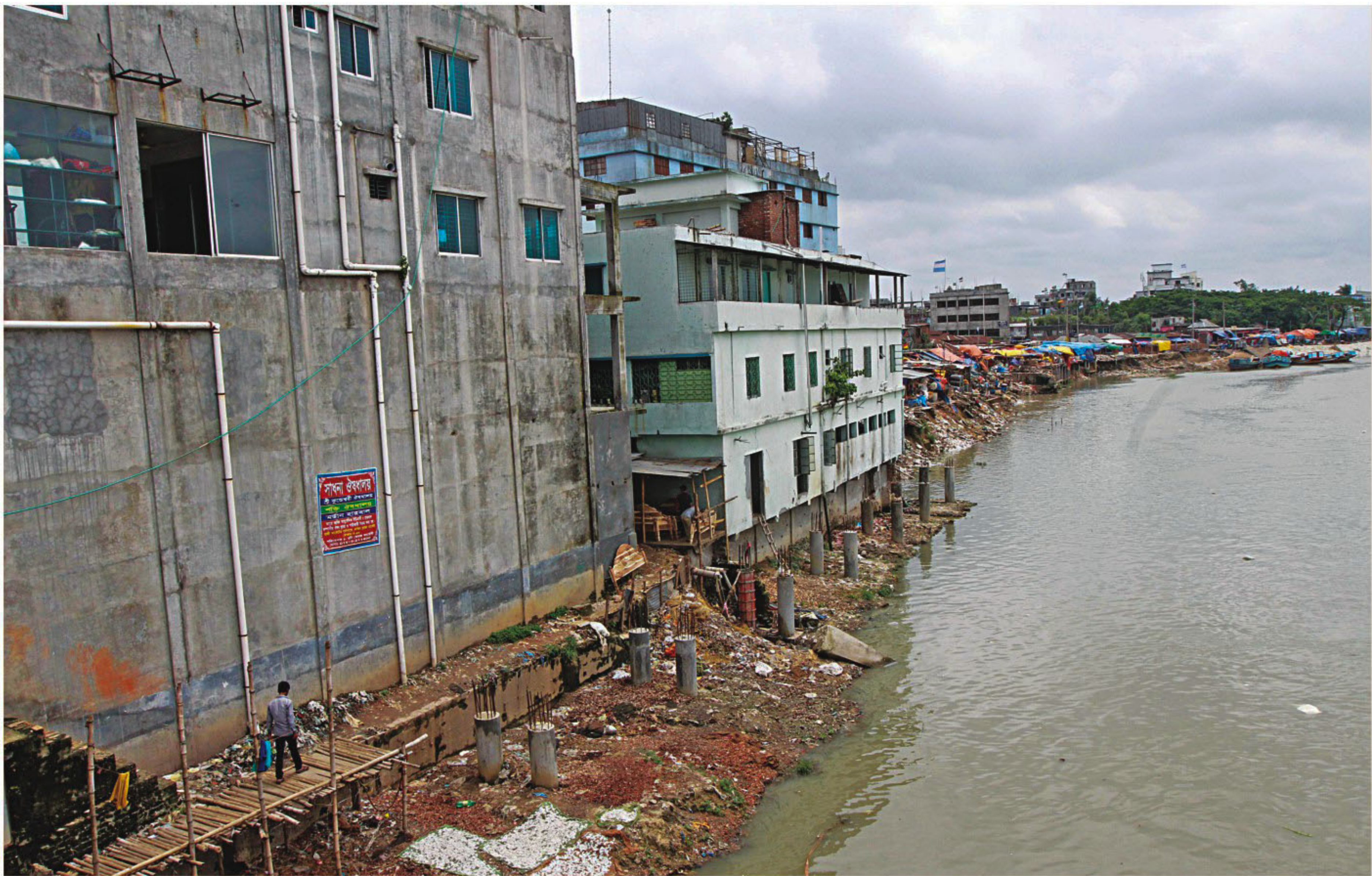
Two commercial buildings of Tongi kitchen market stand within the foreshore of the river Turag. The Gazipur district administration and the BIWTA jointly conducted a drive on May 15 to reclaim the foreshore for a proposed walkway. Around 60 makeshift structures were knocked down by the authorities but the two buildings, built by the market's mosque authorities, remained unscathed. BIWTA officials and the district administration earlier bent the foreshore alignment and set up boundary pillars in the river to save the buildings.
