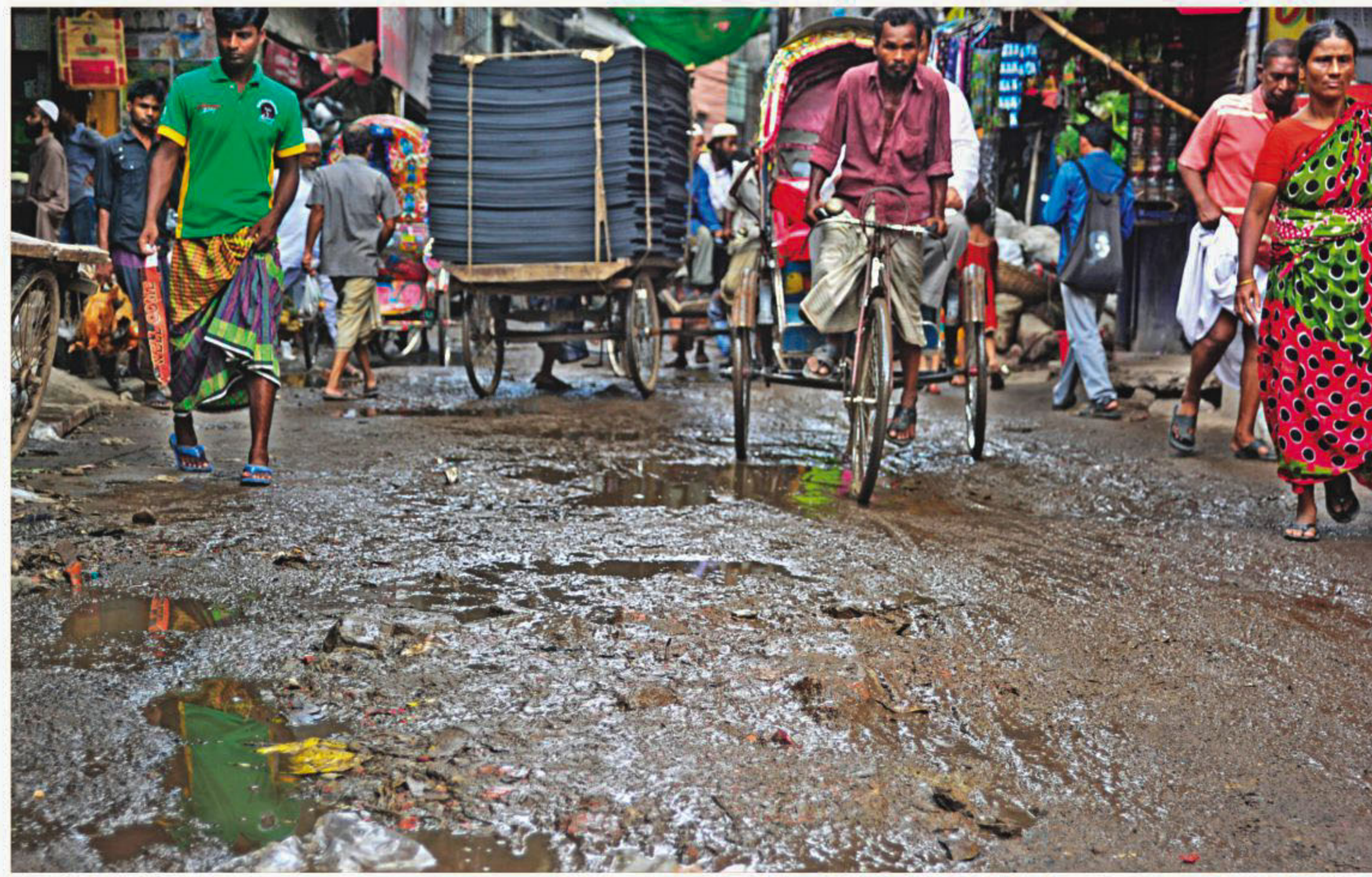
Haji Osman Gani Road in Alu Bazar of old Dhaka has been in this sorry state for the last two years causing immense sufferings to commuters. The photo was taken yesterday.
