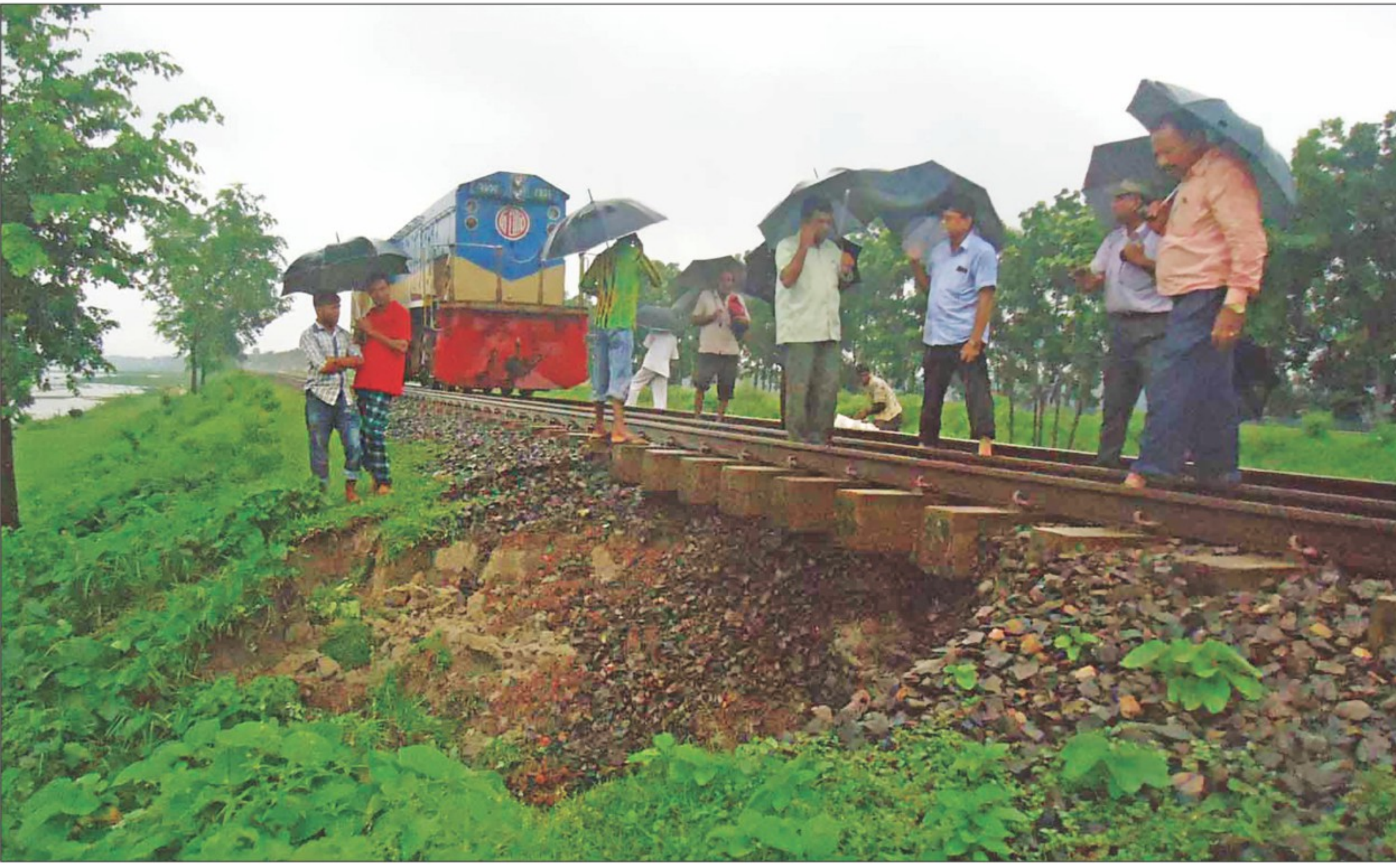
Rail communication between Dhaka and the north and the southwest breaks down yesterday morning after gushing rain water washed away the ground under a rail line in Analiabari of Kalihati in Tangail.
