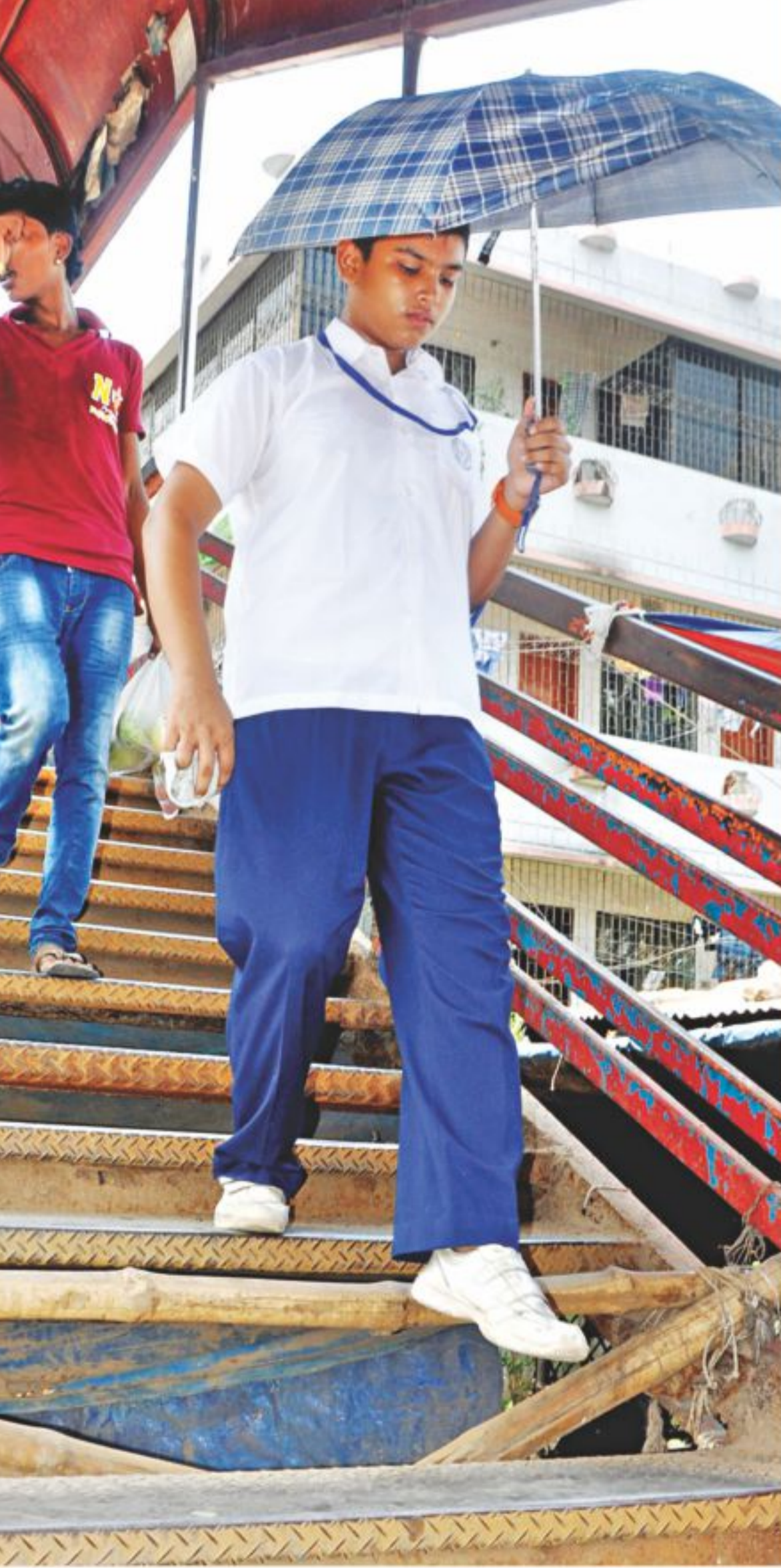
This footbridge in Kamalapur Railway Station area in the capital has been left in this state with several steps missing for a long time while a large number of people, mostly school students, use this every day endangering their lives. The photo was taken on Sunday.
