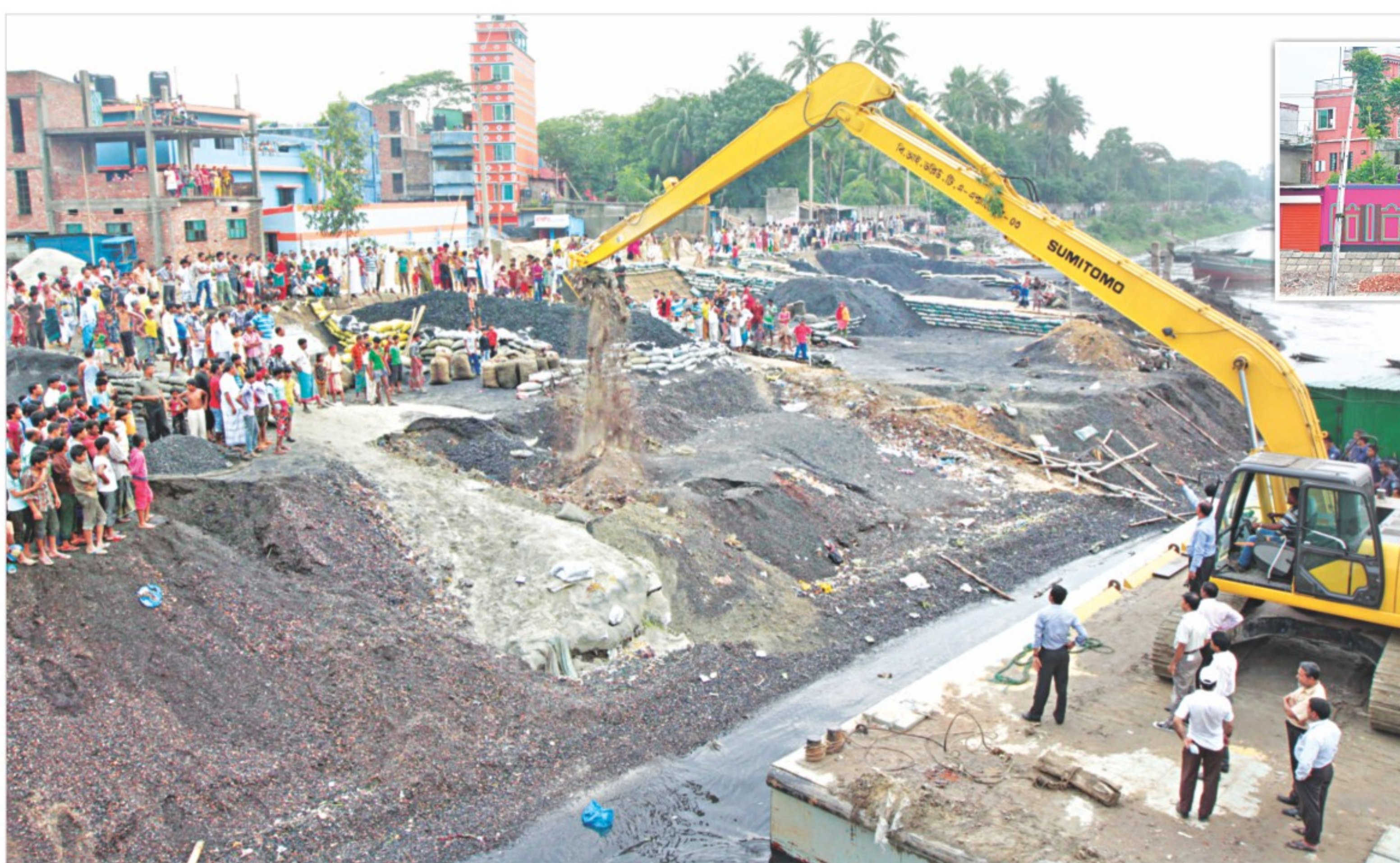
Dhaka district administration and BIWTA in a joint drive demolish illegal structures on the Buriganga near Buriganga Bridge in Postagola yesterday. Workers employed for the joint drive tearing down the walls of a two-storey house, inset.
