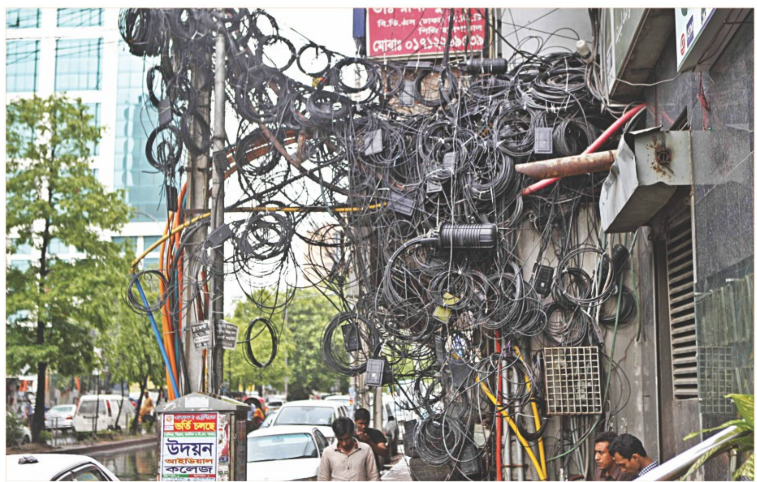
Tangled utility cables hanging dangerously on Bir Uttam AK Kandker Sarak in the capital's Mohakhali almost touching the heads of the passers-by. Repeated publications of such pictures in the media have so far failed to wake the authorities up to put the cables in the right place. The photo was taken recently.
