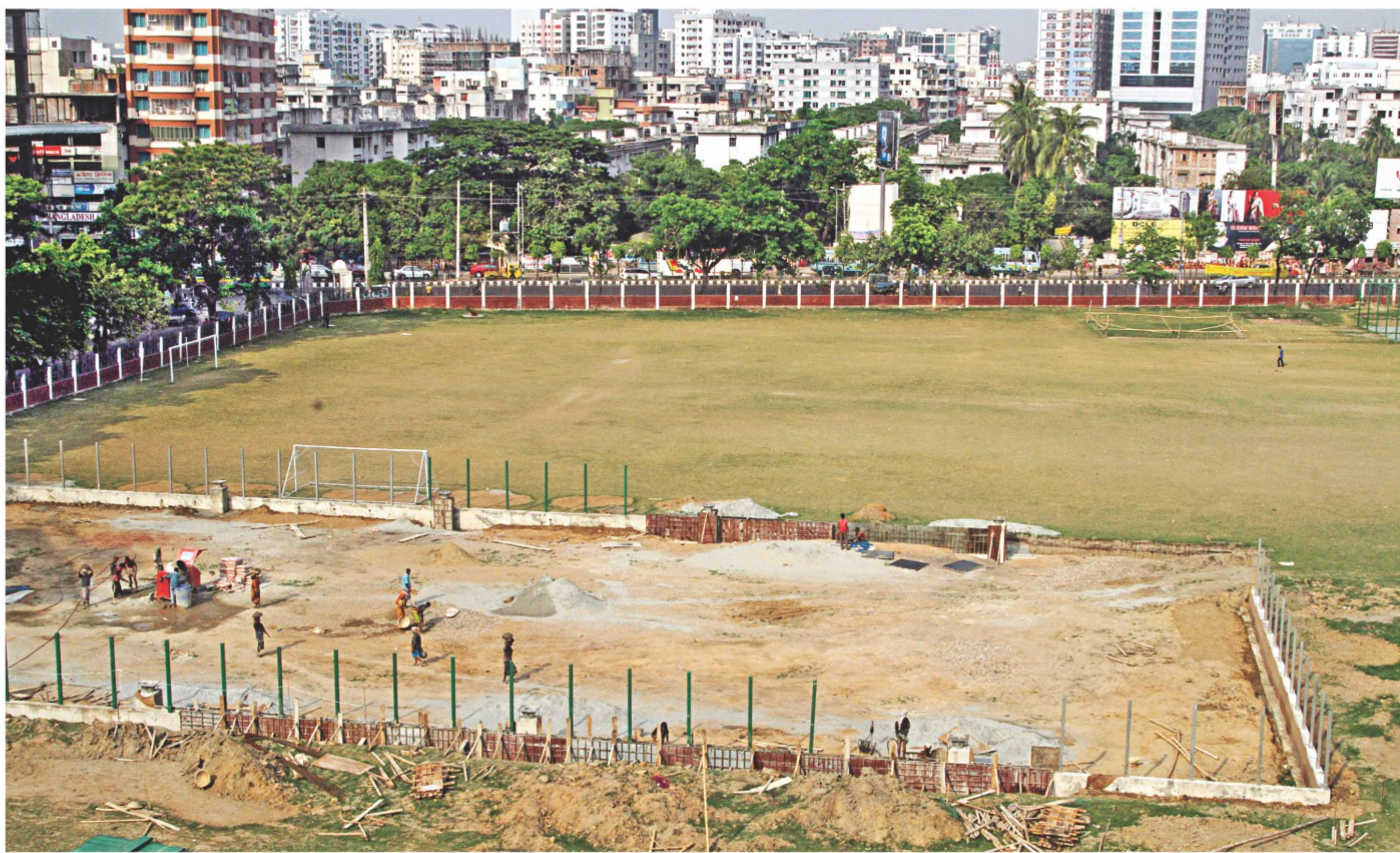
Work continues in full swing day and night to hurriedly build two tennis courts, two badminton courts and a basketball court for a club named after Prime Minister Sheikh Hasina's slain brother Sheikh Jamal, on Dhanmondi road-8 playground. The Local Government Engineering Department is doing the construction for the private club with public money amounting to Tk 1.63 crores. Two writ petitions are currently pending with the High Court to free the playground of illegal occupation. During a hearing on one of the petitions on Sunday, the club's counsel said no construction was taking place at the playground and assured the court no such work would be carried out. PHOTO: STAR
