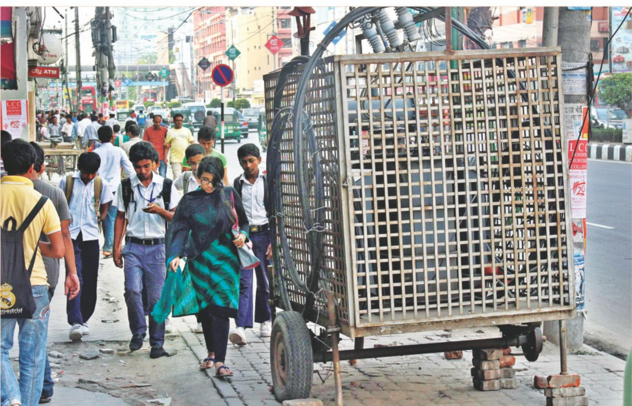
People walk past a power transformer on the footpath beside Kazi Nazrul Islam Avenue in the capital, putting themselves at risk of accident anytime. The transformer was set up on an emergency basis after one atop the electric poles had gone out of order around 20 days ago. The photo was taken recently.
