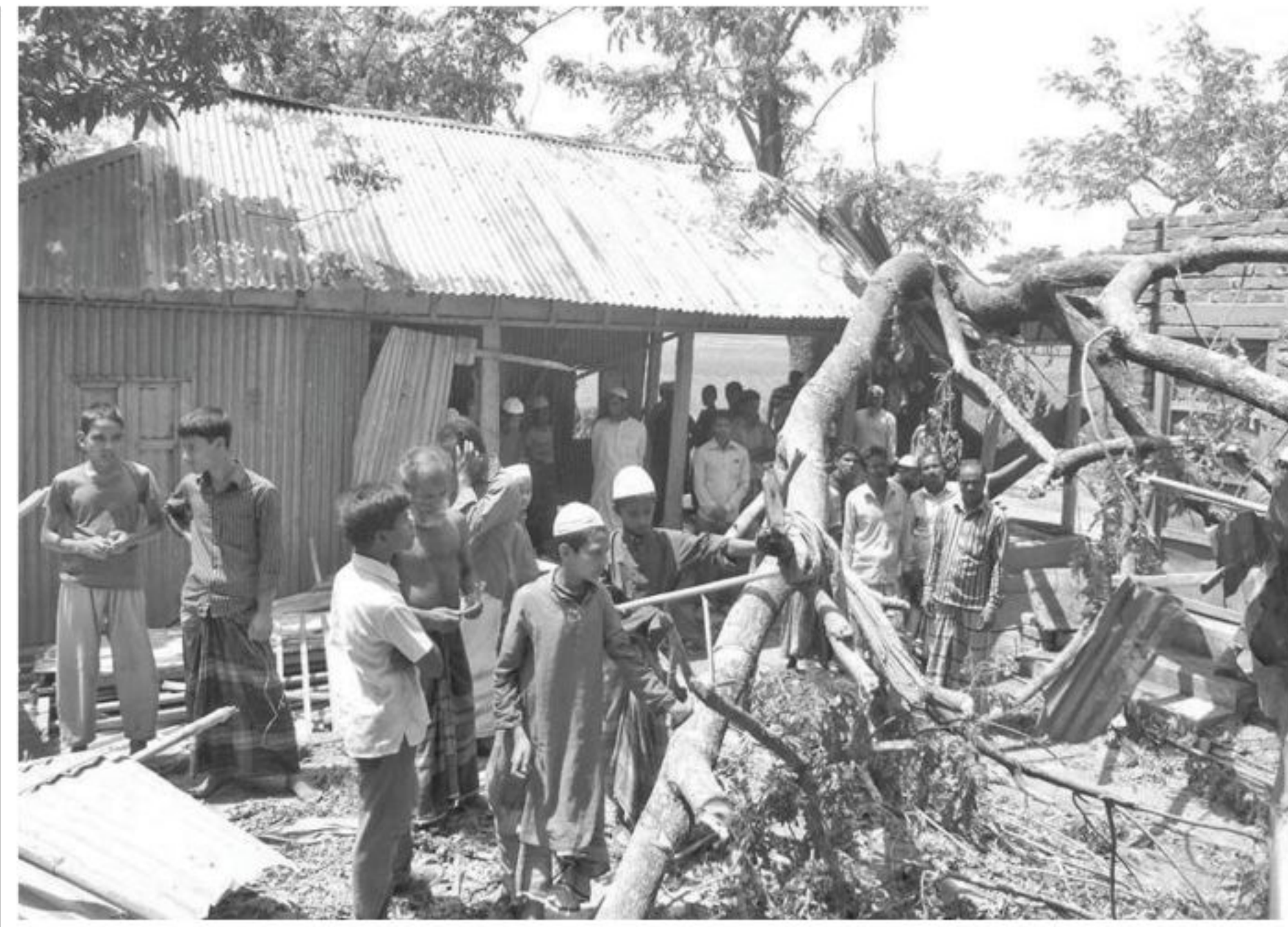
Shahadat Uloom Madrasa at Teroshira village in Gouripur upazila under Mymensingh district lies damaged as a storm lashed the area early yesterday. A resident student of the madrasa met a tragic death and a few others got injured in the incident.
