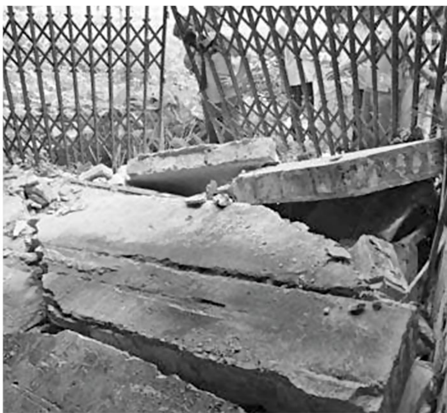
The wall of the canteen of District and Sessions Judge's Court in Munshiganj town collapsed yesterday noon, leaving two lawyers seriously injured.
