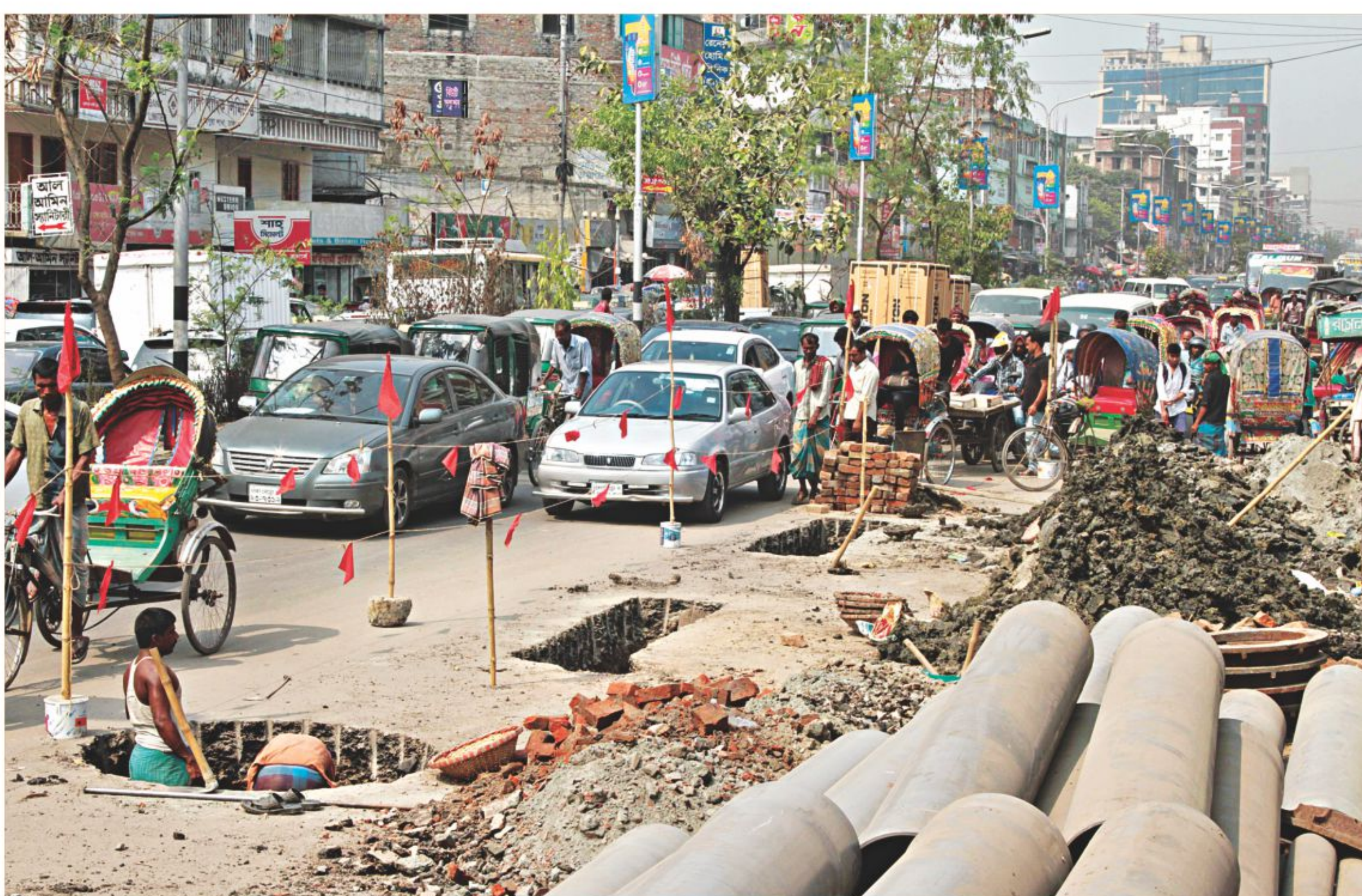
Dhaka Wasa digging a portion of DIT Road in the capital's Rampura for installing a sewerage pipe during the middle of the day when the traffic is heaviest, creating a long tailback on one of the major roads yesterday, first day of the HSC exams. The road has been narrowed to almost half its size at a time when thousands of examinees need to commute for reaching exam centres on time.
